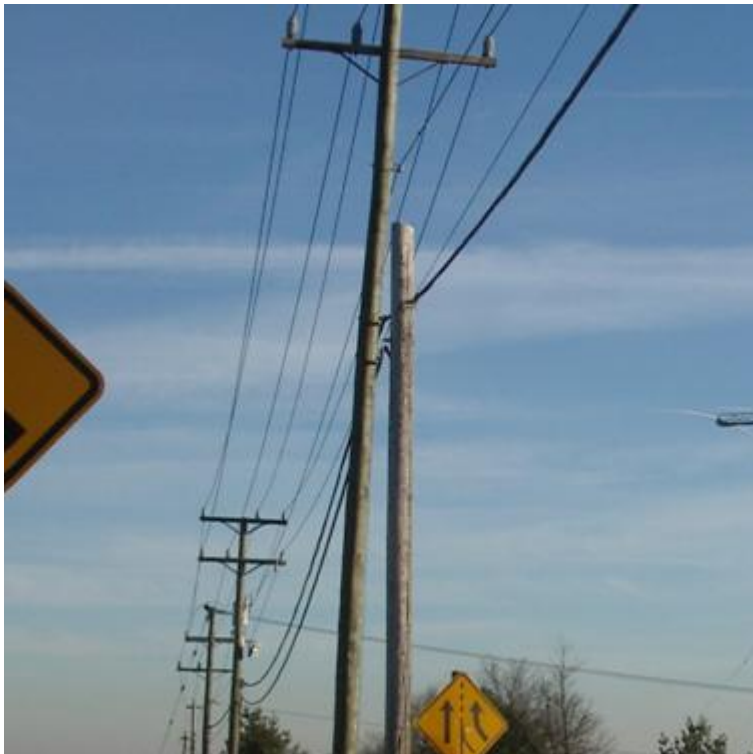
Figure 2-43: Stacked 3-phase power line conductors
