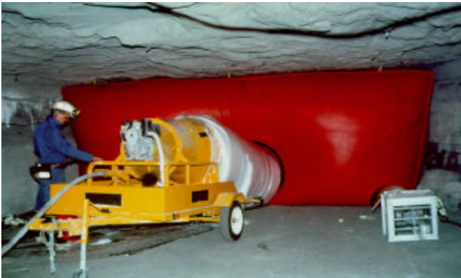
Example of a foam generator in use
