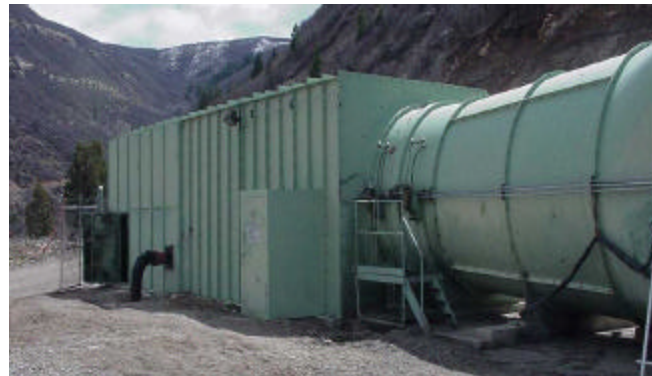
Typical mine fan installation
