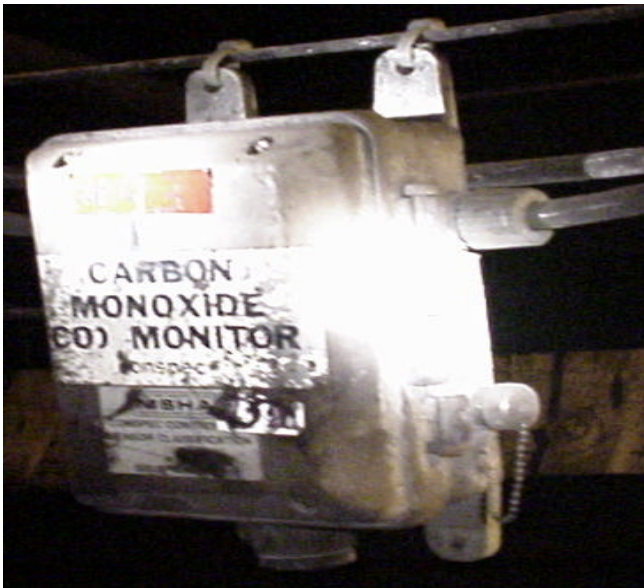
Example carbon monoxide sensor installation
