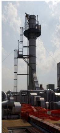
Large Roof Top Fan
