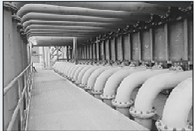
Water (top) and sorbent recycle (bottom) injection lines above absorber grid packing
