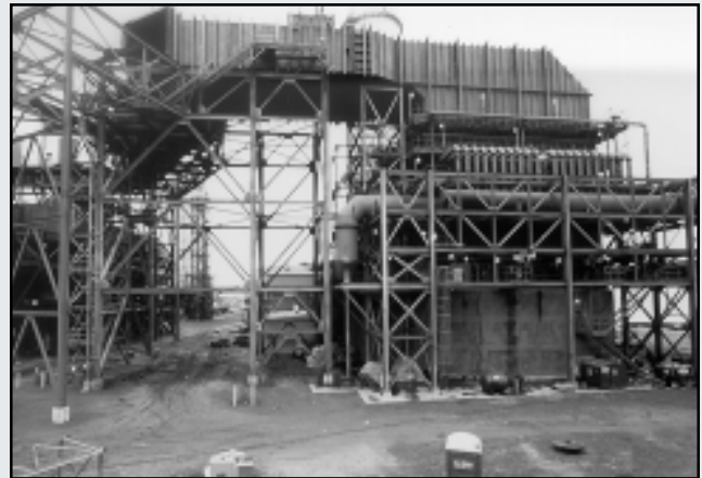
Absorber module with flue gas inlet ductwork and process water and sorbent slurry lines
