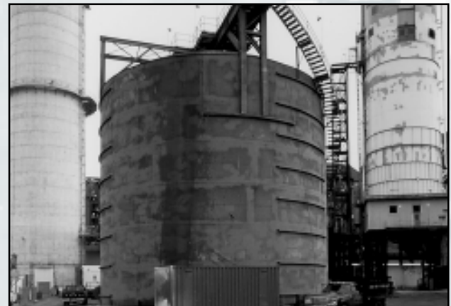
One million gallon gypsum storage silo with flyash hopper (right) and stack (left)
