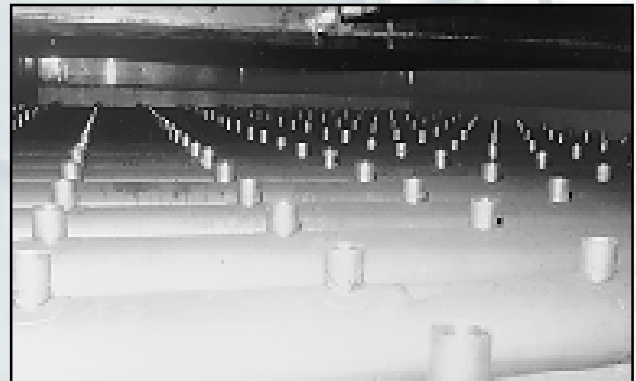
Sorbent recycle injection system inside absorber module
