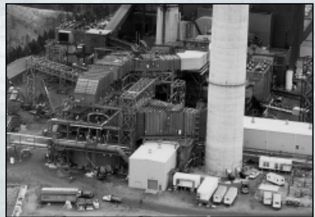
Interconnection of absorber module and stack
