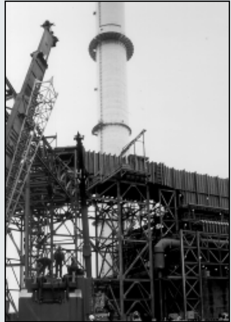
Ductwork being installed with stack in the background and absorber module in lower right corner
