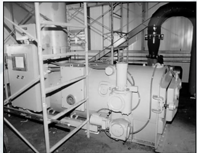
New coal feeder for Coal Reburning system
