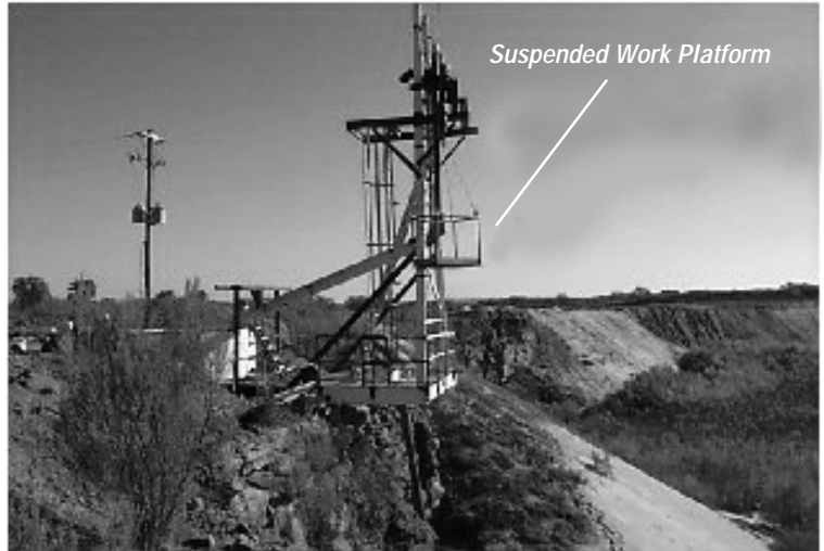
Use a work platform approved by a qualified engineer
