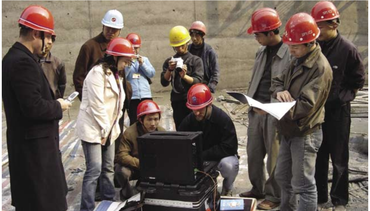
A group of engineers gathers to collect temperature data using the SensorTran 5100 on the Yu River dam construction project in the Guizhou Province of China.
