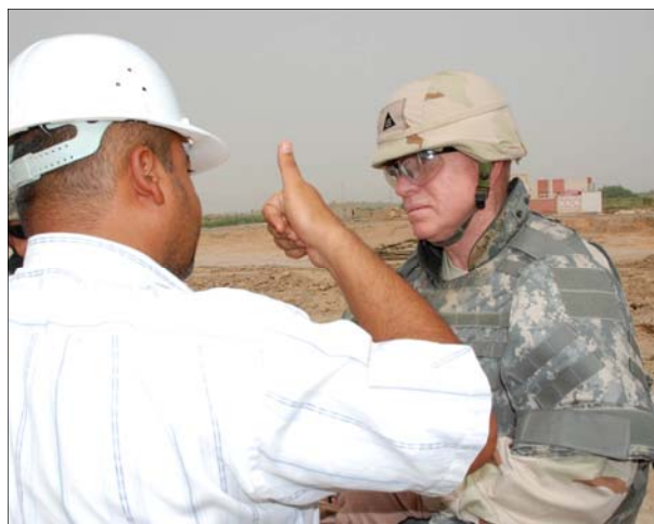
Construction Representative John Biltoft with Gulf Region Division and Iraqi civil engineer Alaa discuss the current progress of a $749,000 water treatment plant being built in northern Dhi Qar Province. (USACE photo by Norris Jones)
