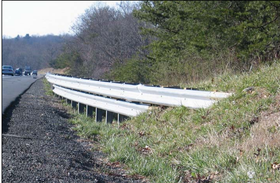
Figure 3.15: W-Beam Buried in Backslope
