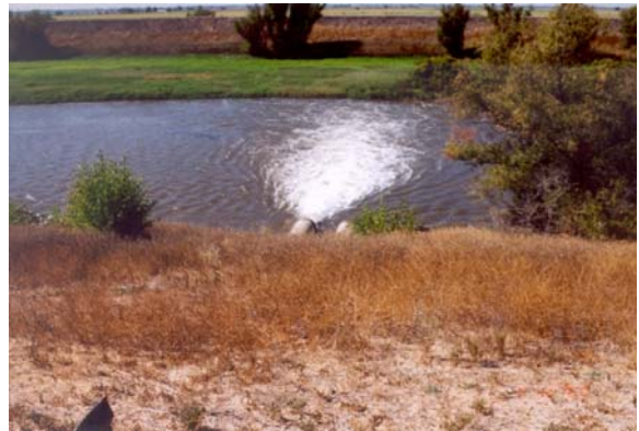
RD 1000 Pumping Plant 4 Discharge to the Natomas Cross Canal
