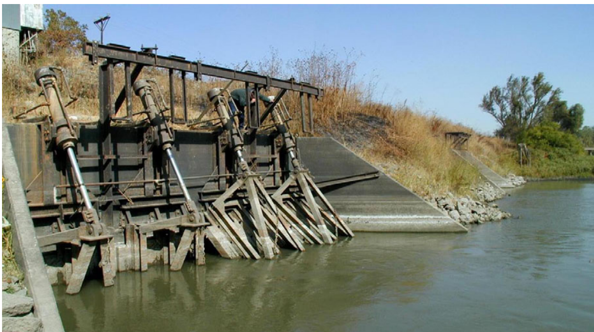
Discharge of Pumping Plant No. 3 into the Sutter Bypass
