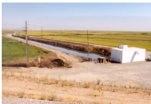
RD 1000 Pumping Plant 4
