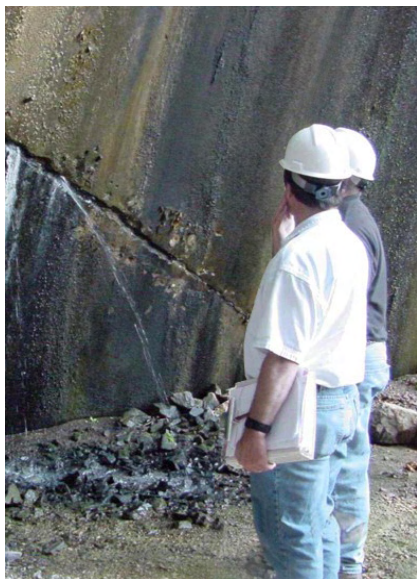
Timely inspections and maintenance help ensure that Reclamation continues to meet the needs of the American public.
