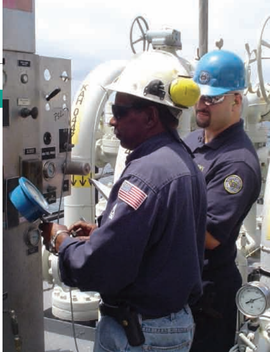
An MMS inspector witnesses testing of a safety device at an instrumentation panel.
