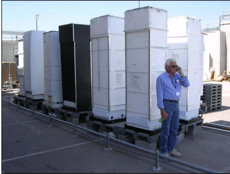
Figure 19. Standardized towers from L'eau.
