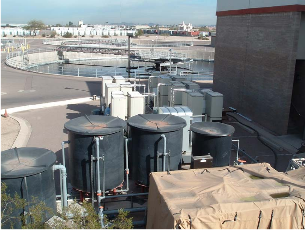
Figure 7. Towers installed at pilot site with generator, tanks, and tactical water purification system.
