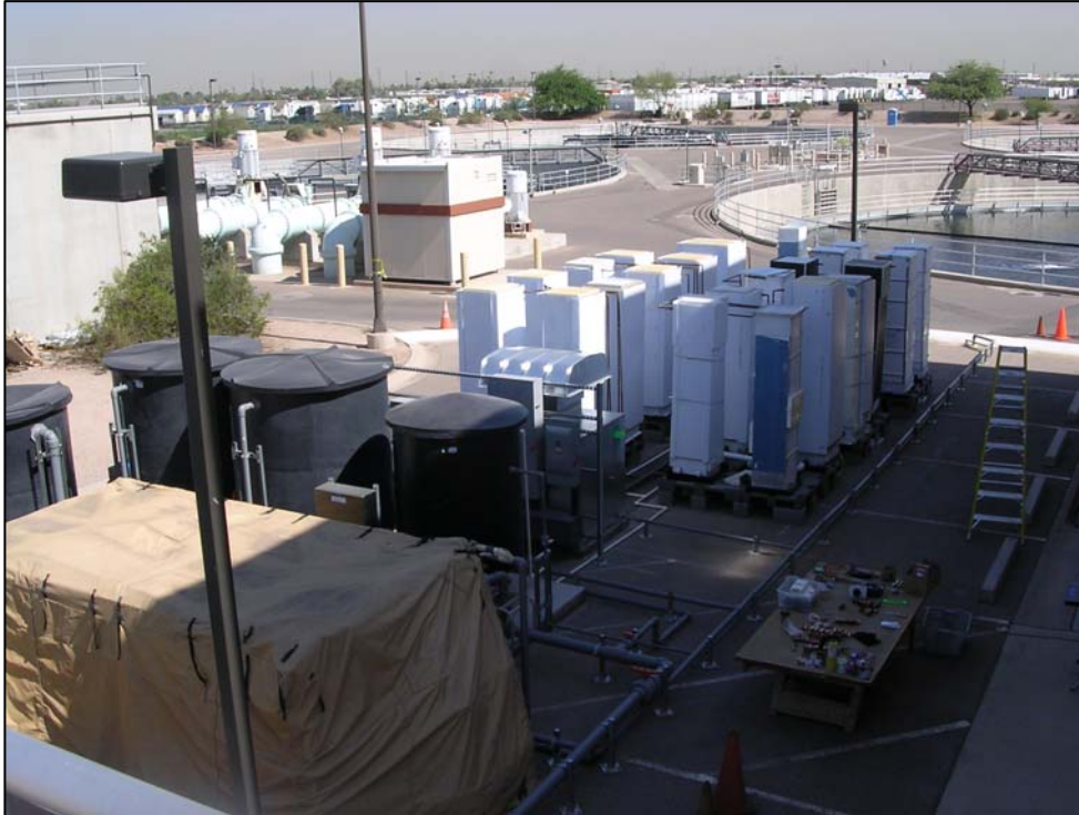
Figure 16. Overview picture of the as-built pilot plant.
