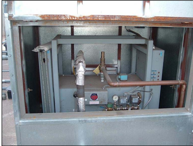
Figure 18. Electric steam boiler in its enclosure.
