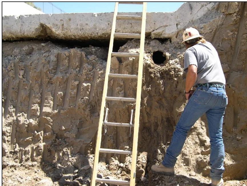
Figure 3. —Undermining of the chute slab has occurred due to flow entering at joints and cracks and transporting foundation material through unfiltered drains.
