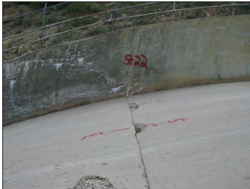
Figure 1. —Initial damage due to uplift generally occurs at the construction joints.
