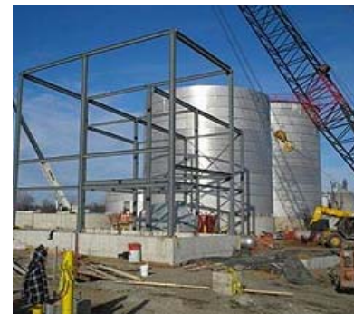
Ethanol plant under construction in Albert City, Iowa (~100 million gallons of ethanol per year).
