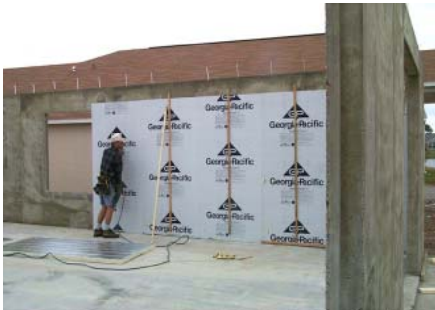
Figure II-15. Eight-foot-long panels of insulation being applied over 9-ft-high poured walls, held in place by strapping. In production, there was little or no extra cost for 9-ft-long insulation. (The roof in the picture belongs to the adjacent house.)
