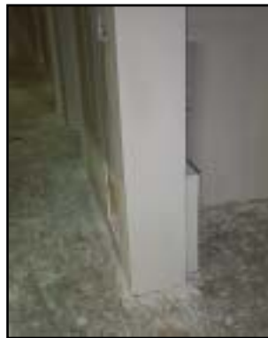
Figure I-50. Central Return in Hall
