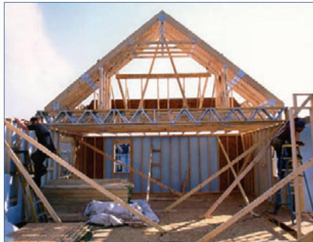
Advanced framing helps to save building materials and construction costs and create more room for insulation, making the house more energy efficient.
