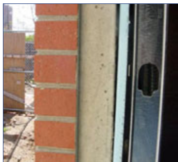
Wall construction consisted of 6 inch and 8 inch concrete panels, backed with half-inch expanded polystyrene foam insulation, steel framing, and R-11, faced, fiberglass wall cavity insulation.
