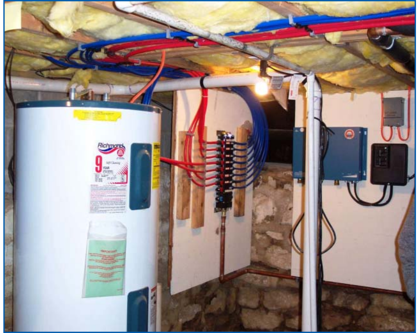
Hot water system in cottage
