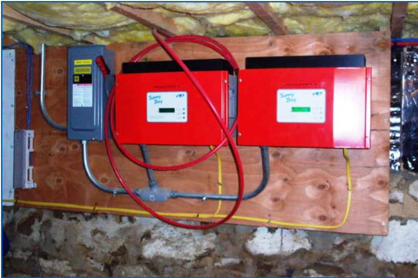
PV system inverters
