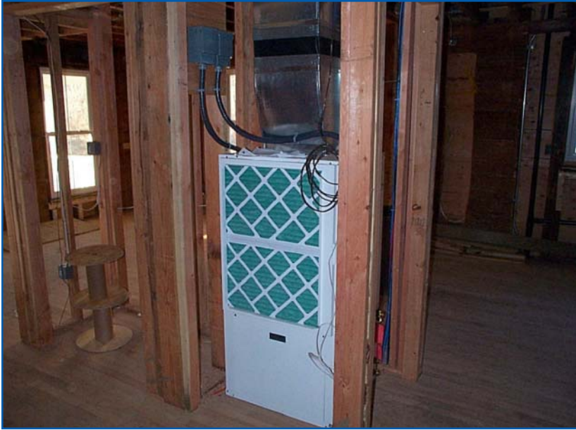
Ground source heat pump in conditioned space
