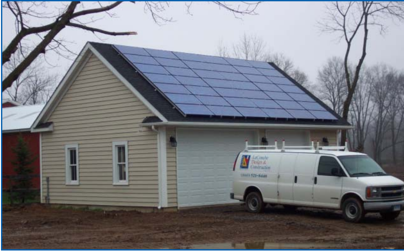
Garage PV system for Cottage home
