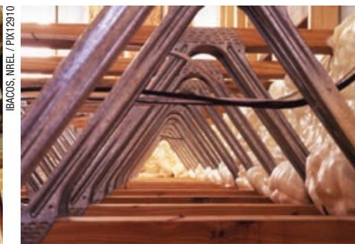
Open web trusses provide space within the building enclosure to run electrical wires and ducts.
