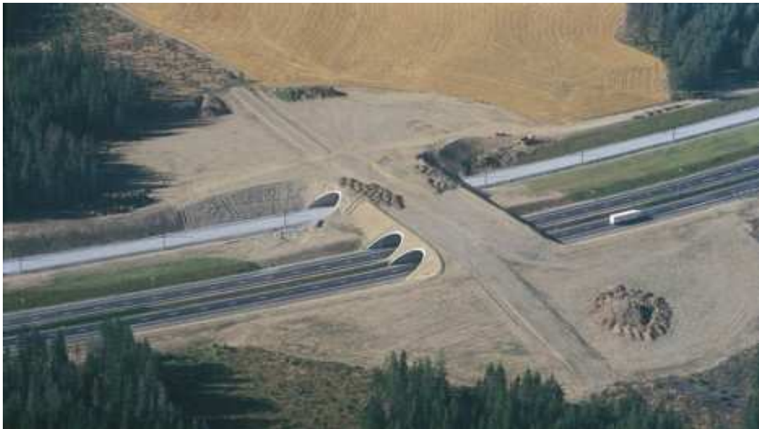
Fig.9-View of Combined Overpass under Construction on Rail line and Road in Europe
