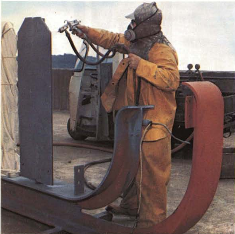
New space paint is applied to girder of Golden Gate Bridge to test its resistance to salt spray and weathering. The inorganic paint requires only one coat and is expected to last twice as long as conventional paints.
