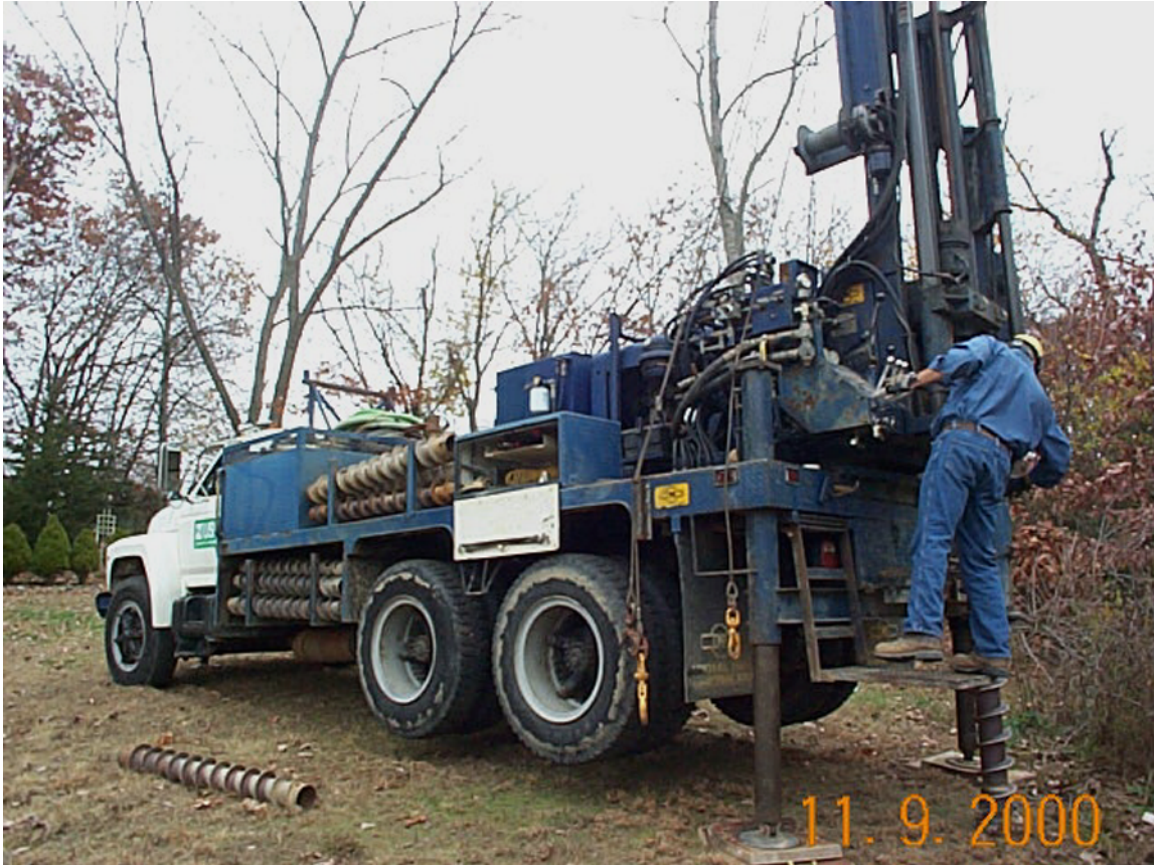
USGS drill rig installs land-based portion of pond-level monitoring gage on Kingsbury Pond near Franklin, MA. (photo by J. L. Zanca)
