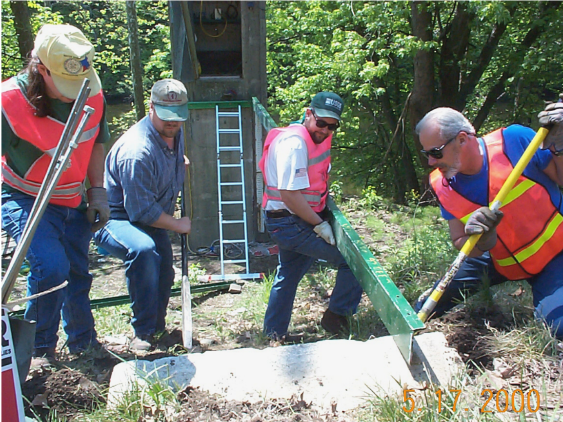
Massachusetts Data Section staff install new walkway to gage house on Westfield River at Westfield, MA, 01183500. (photo by T.R. Driskell)
