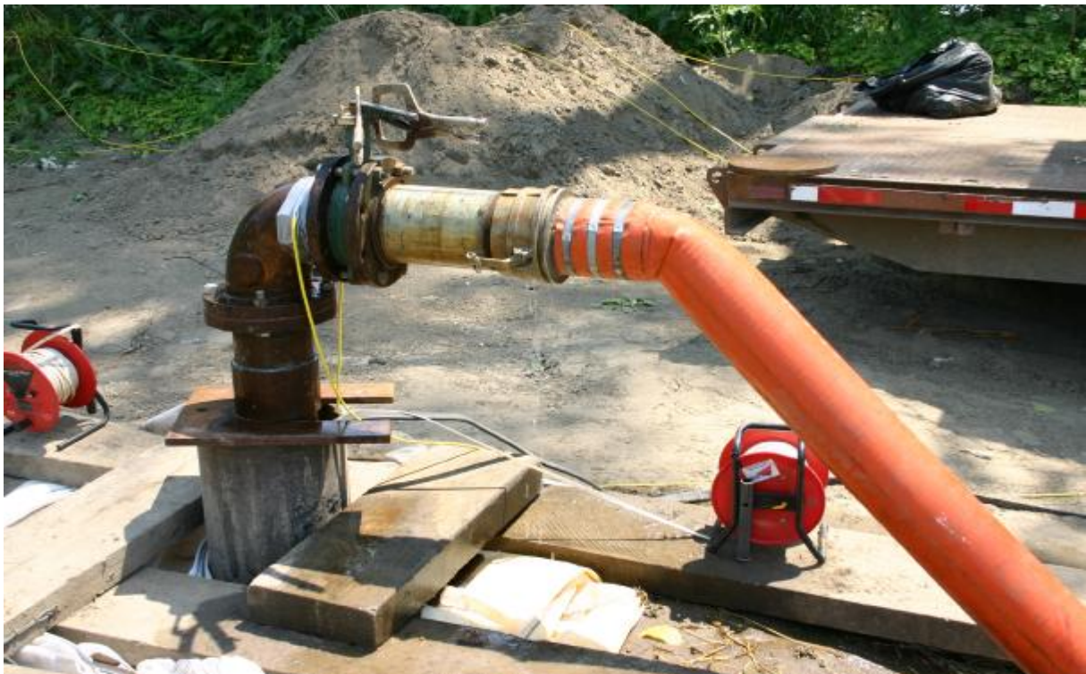
Top of the test pumping well.
