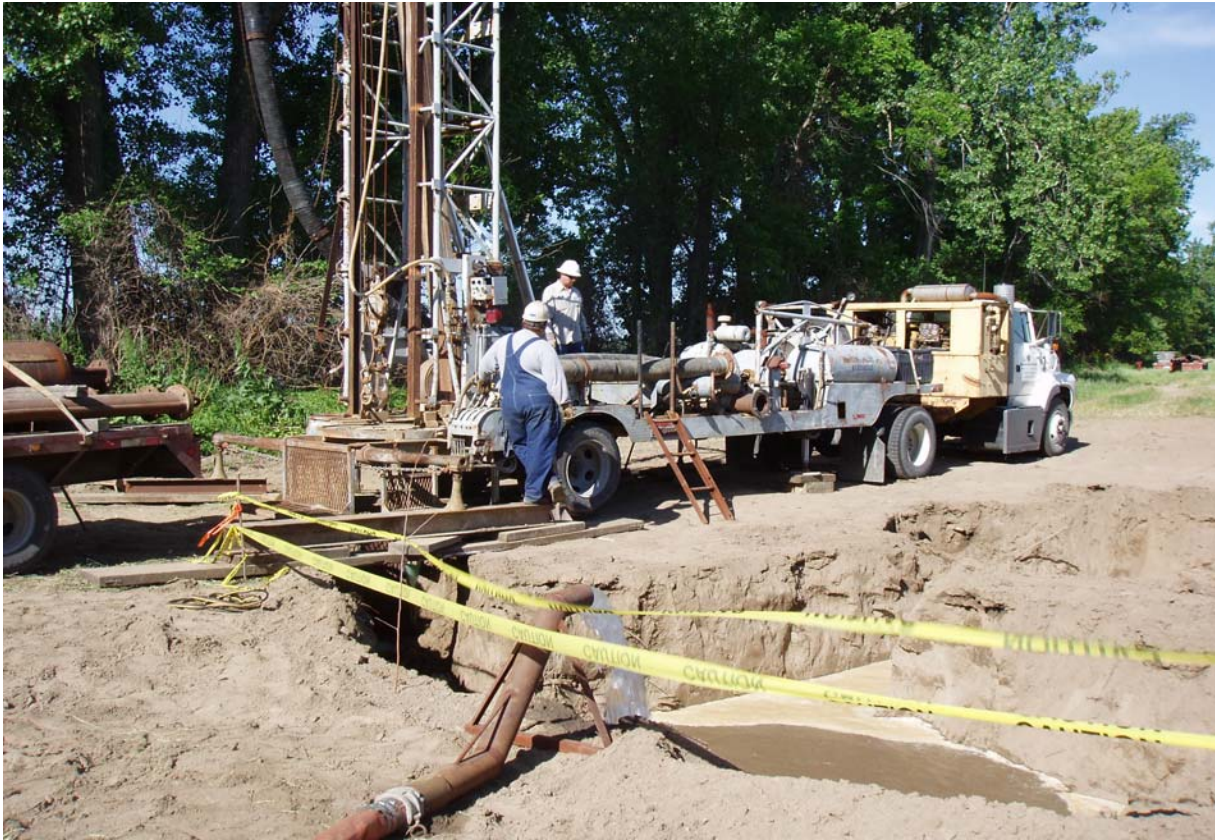
Reverse rotary drilling rig set up to drill the test pumping well.
