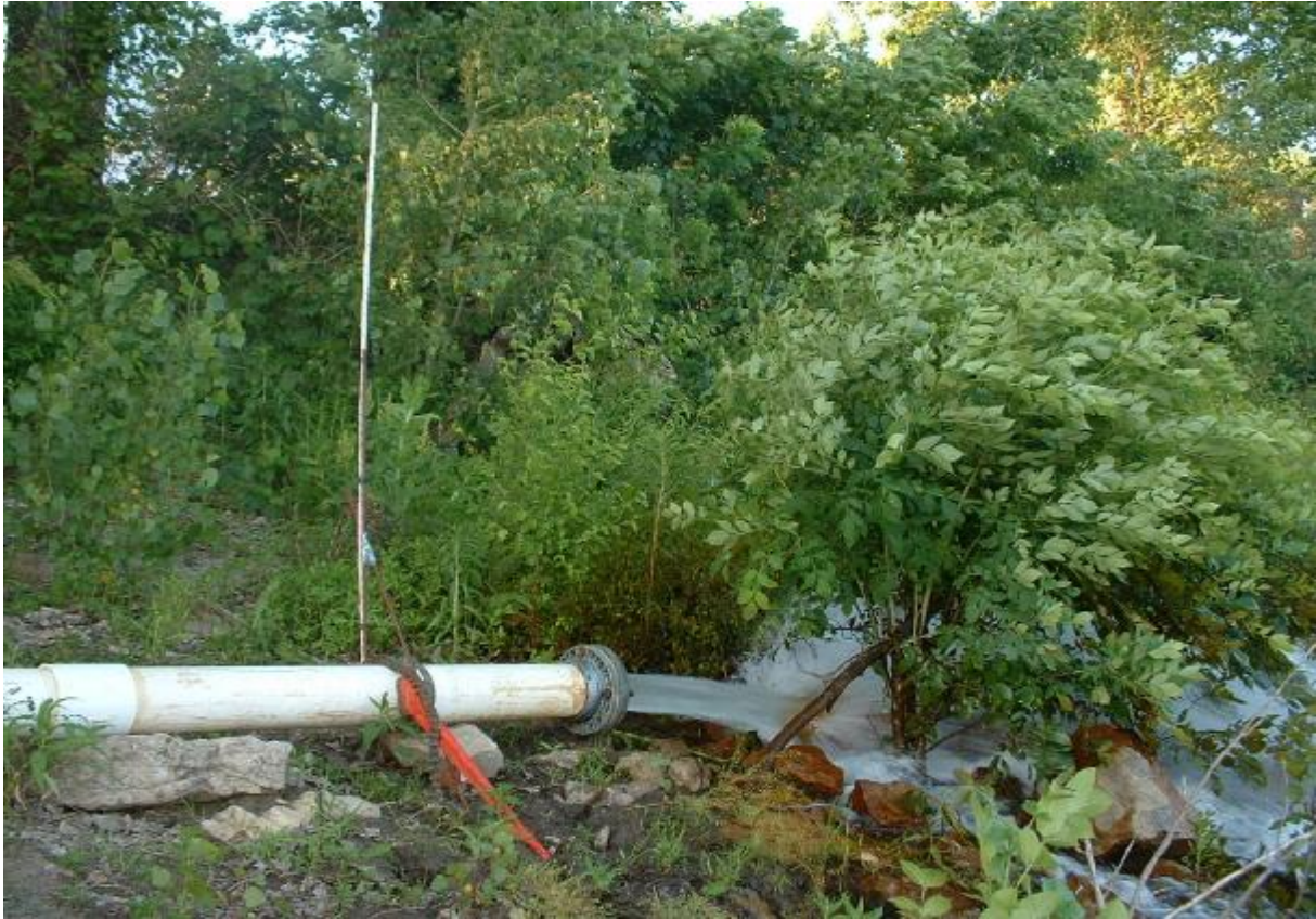
Orifice weir used to measure the pumping rate for the aquifer pumping test.
