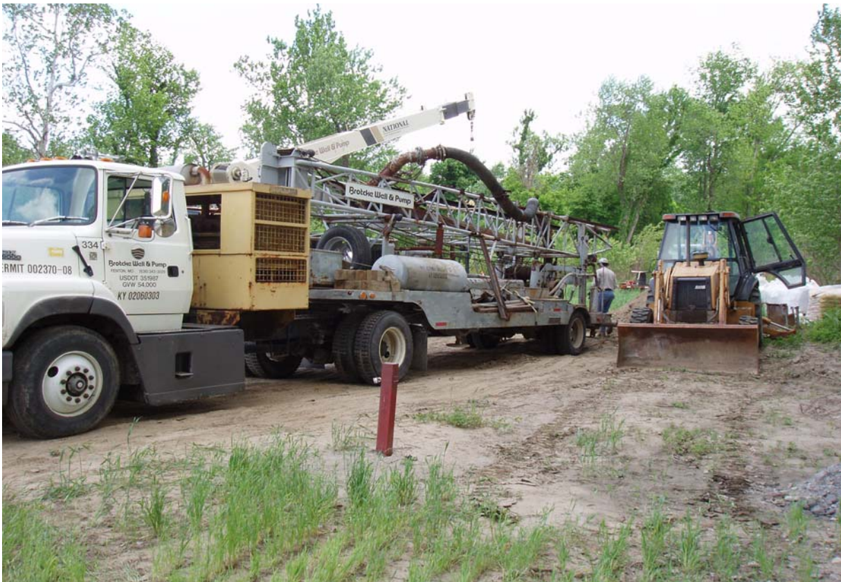
Setting up the reverse rotary drilling rig at the test pumping site.
