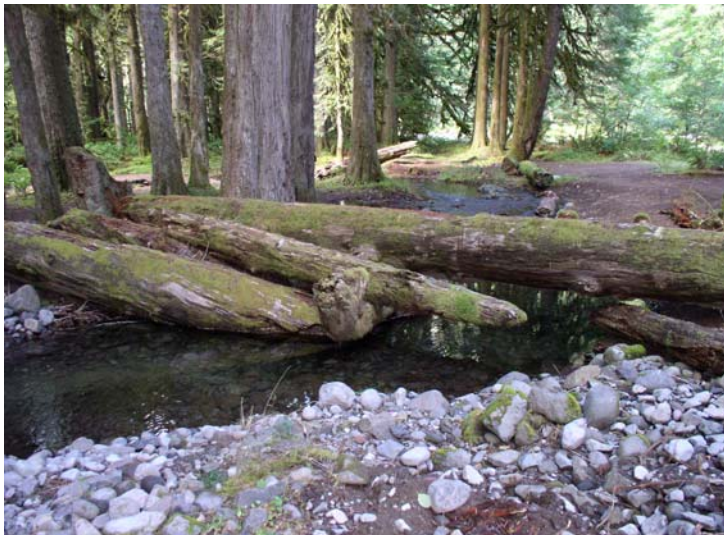
Photo below left: The completed project. When flows increase during winter storms, the large wood provides shelter and refuge for young salmon.
