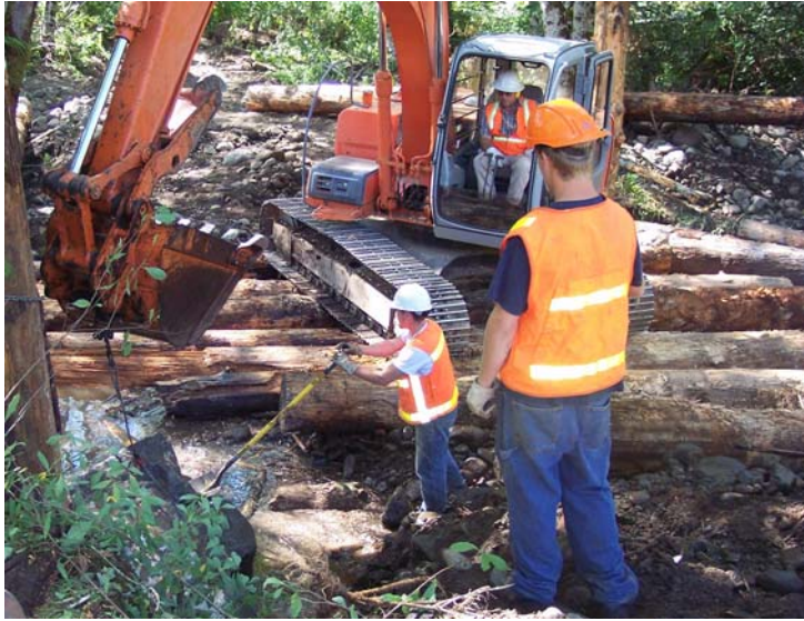
Photo above left: Workers direct placement of logs and boulders to restore habitat elements in a side channel.
