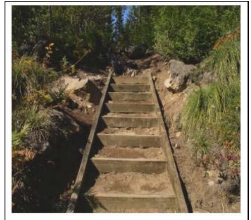
Photo above right: Shows an access trail to the lake eroding with sediment entering the lake. Photo below right: Shows the same area after construction of steps designed to reduce erosion to the lake.
