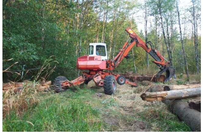
Photo above: Salmon habitat restoration on private lands can be funded through Payco. Here a walking spider backhoe reconstructs an old beaver pond.
