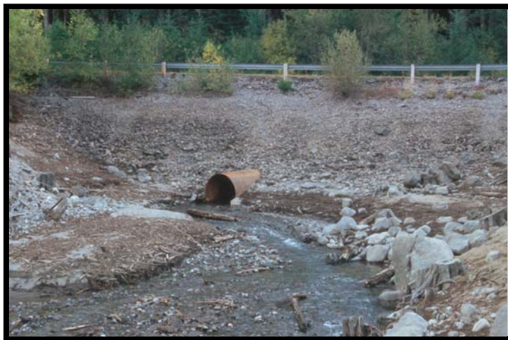
View of Pinnacle Creek with old culvert. About 2,500 cubic yards of fill was removed to restore the stream channel.
