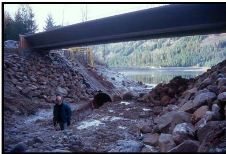
Engineers prepare to pull what remains of the 130 foot culvert. Laurance Lake is in the background. Bull trout now may freely access Pinnacle Creek at all lake levels, which fluctuates up to 8-10 feet depending on downstream water needs. The new streambanks were planted with native grass seed.
