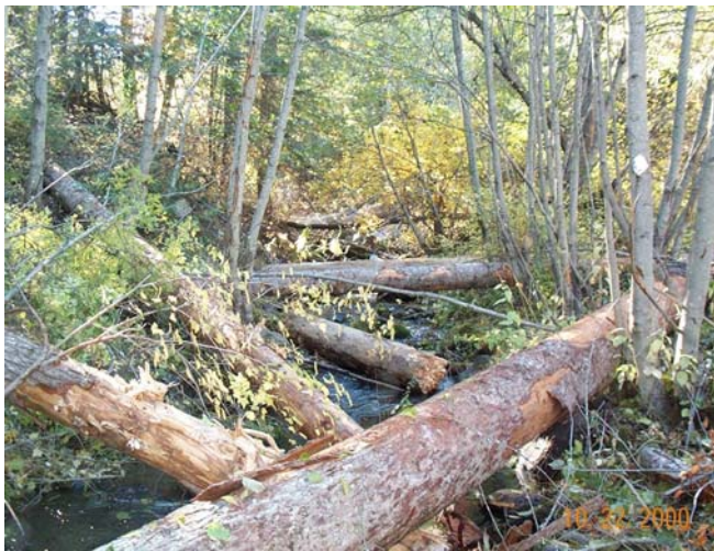
The newly restored channel is loaded with large wood for fish habitat.
