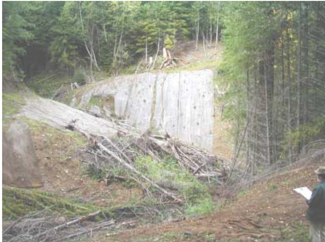
Figure 18. Steep stream banks and road ditch runoff resulted in poor erosion matting effectiveness at one stream crossing on Road 2586.
