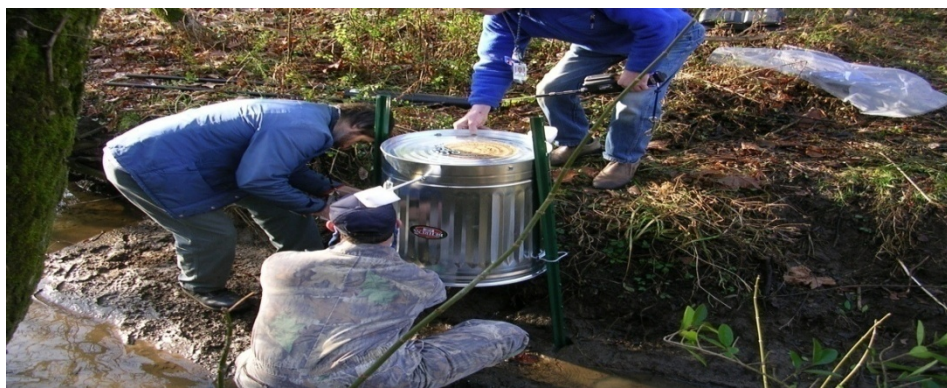
Figure 2: Installation of PID Ambient Air Apparatus
