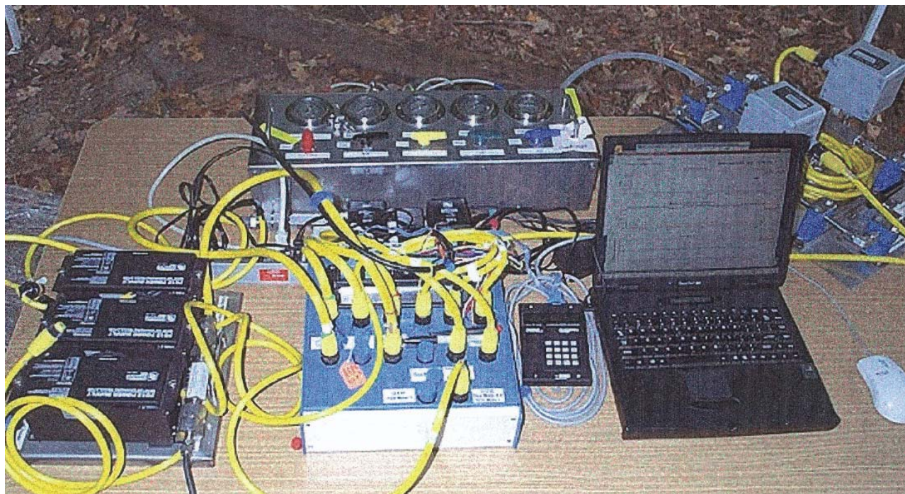
Figure 32. Photograph of a laptop computer connected to the Campbell Scientific CR23X Data Logger on the data-acquisition panel of the Multifunction BAT 3 .
