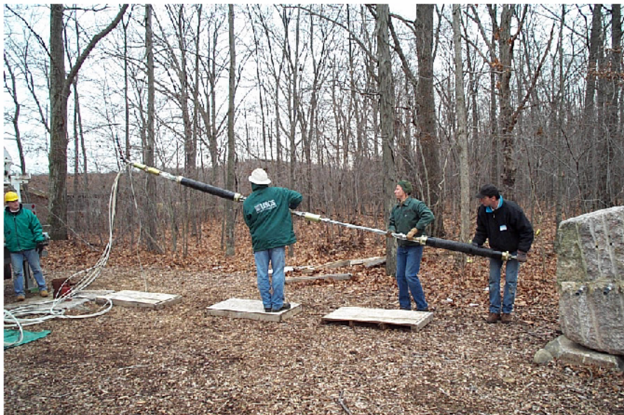
Figure 47. Photograph (courtesy of John Jaacks) of the support needed while raising the downhole components of the Multifunction BAT 3 off the ground in preparation of lowering it into a borehole.
