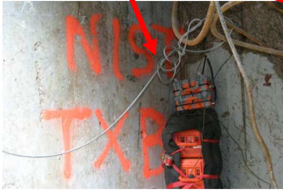
Cable near transmitters
