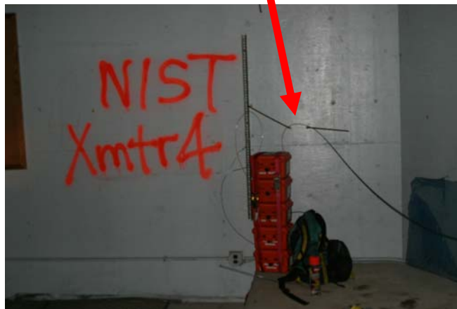
Figure 22. Cable on northwest side of the convention center. This cable was run from the transmitter site (TX 4) to the outside of the building structure.
