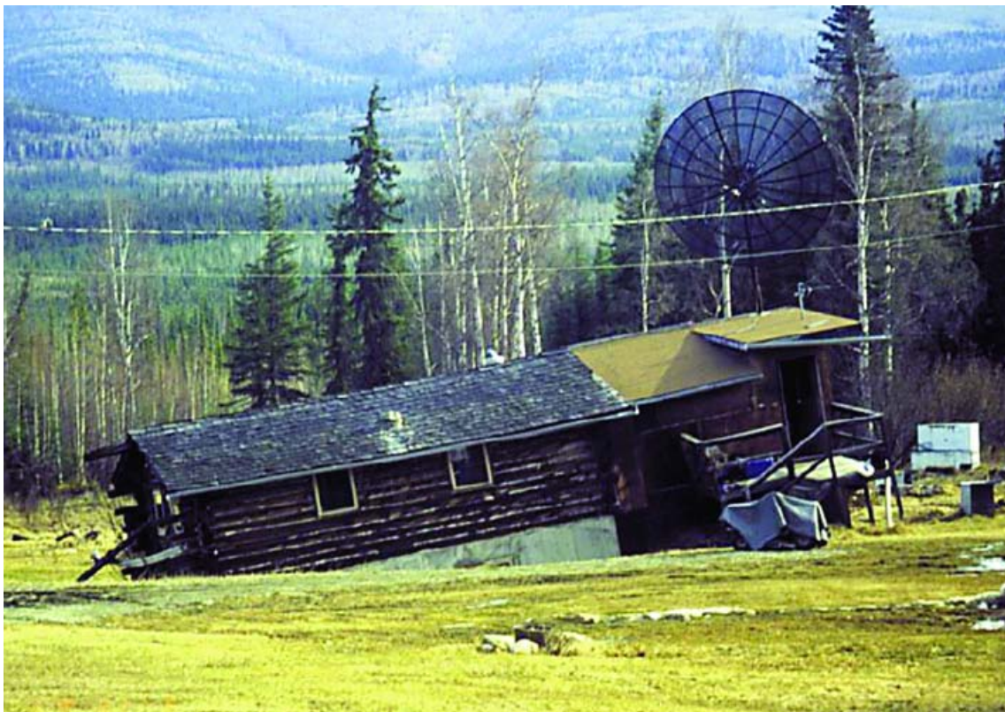
Figure 18: Melting permafrost severely impacts buildings (Source: Larry Hinzman; reprinted with permission)
