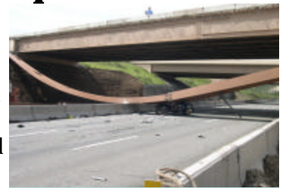
The girder collapse on I-70 in Golden, Colorado
