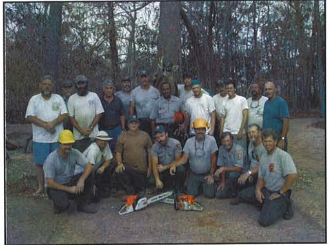
The Southeast Saw Crew removed hazardous trees at the Gulf Islands National Seashore campground to create a useable area to house displaced NPS and Coast Guard employees and their families.
