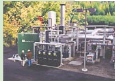
Fuel cell power plant being tested in Connecticut
