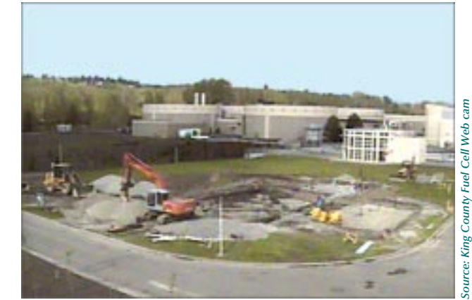
Fuel Cell Demonstration Project Site at the South Treatment Plant
