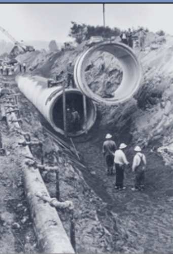
King County has a vast network of underground pipes.
