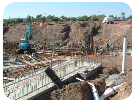
Early work on the TCA, such as pouring footings and installing utilities, has been underground.
