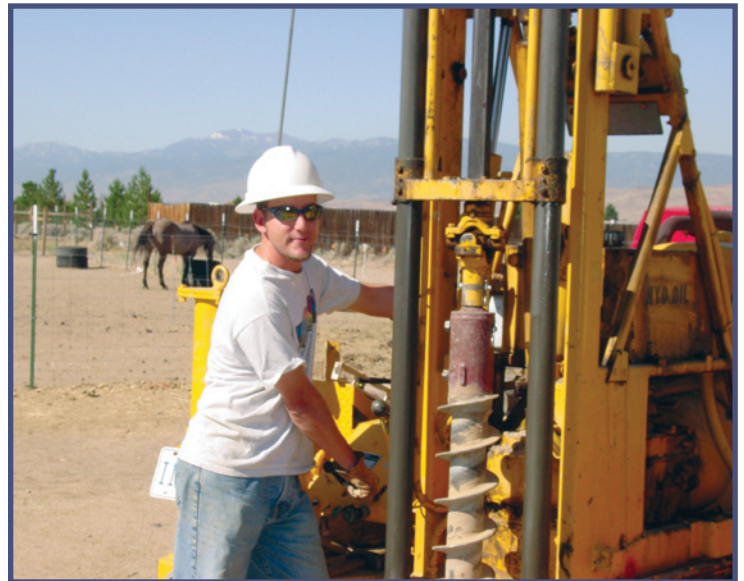
Drilling to place lysimeters at Site D, Spanish Springs Valley. Photograph by Don Schaefer, USGS.
