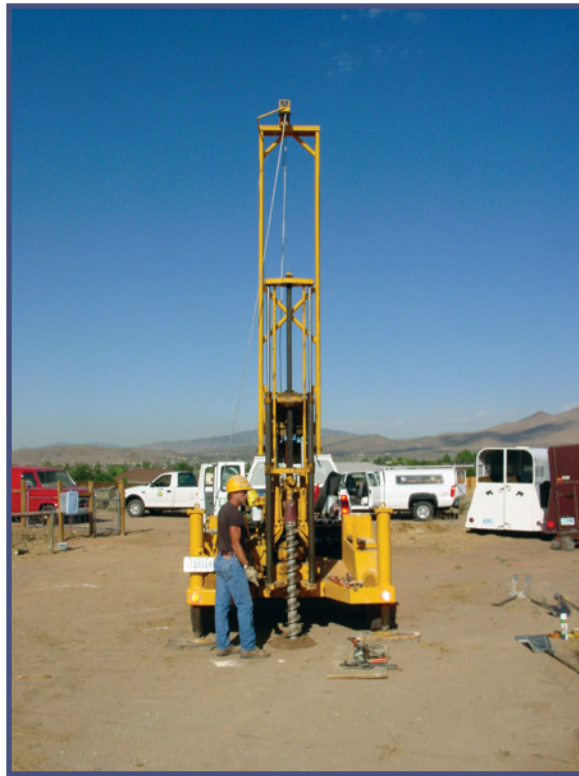
Drilling to place lysimeters at Site D, Spanish Springs Valley. Photograph by Don Schaefer, USGS.
