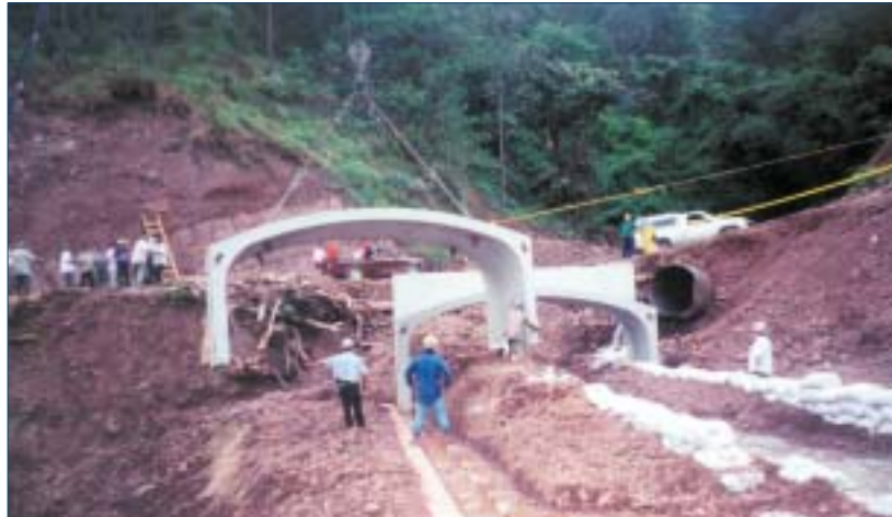
A large mobile crane transfers the bridge units from the trucks to their final position on the base slab.
