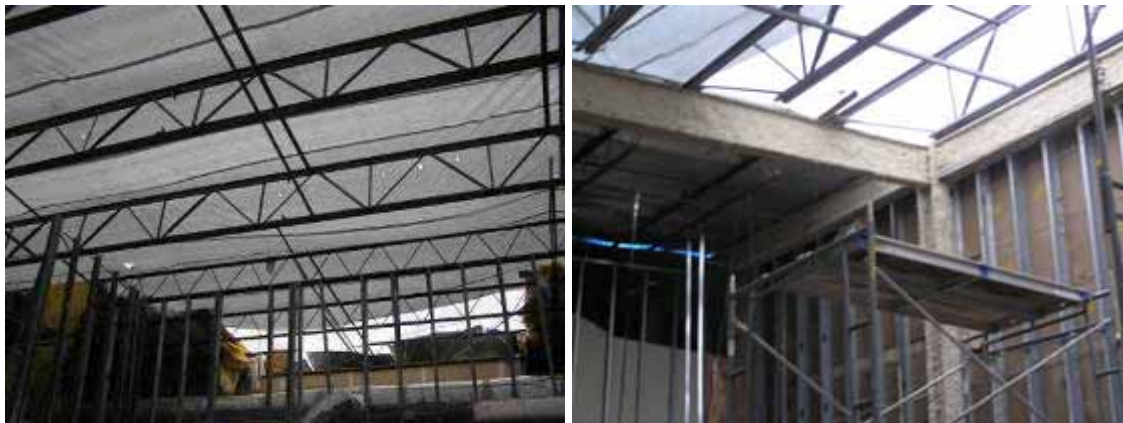
Figure 3-35 Loss of open-web roof trusses and metal-paneled roof deck at Anderson Elementary School in Orange, TX. Note the pictures show the replacement trusses and the temporary plastic covering (Photo credit: NIST).
