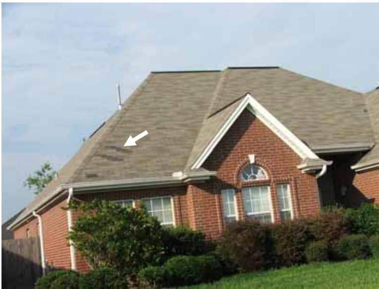
Figure 5-21 Limited damage (arrow) to relatively new three-tab asphalt shingles in Port Arthur, TX. (Photo credit: Dominic Sims, International Code Council)
