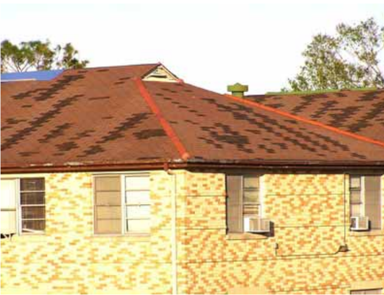
Figure 5-22 Damage to older three-tab asphalt shingles wherein approximately 40 percent to 50 percent of the shingles were blown off the front side of the home in New Orleans. Note the vertical strips of blown-off shingles. This failure pattern is associated with applying the shingles in a process known as “racking” in which shingle are applied vertically or straight up the roof. Racked–applied shingles are susceptible to blow-off as illustrated here, and the process should not be carried out in regions susceptible to high winds. (Photo credit: Robb Smith, Amtech Roofing Consultants)
