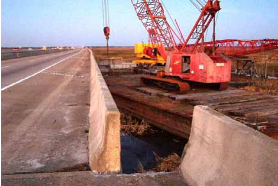
Figure 4-49 US-90 bridge over Pascagoula River with displaced spans due to barge's impact (photo credit: MSDOT, provided by J. O'Connor, MCEER)
