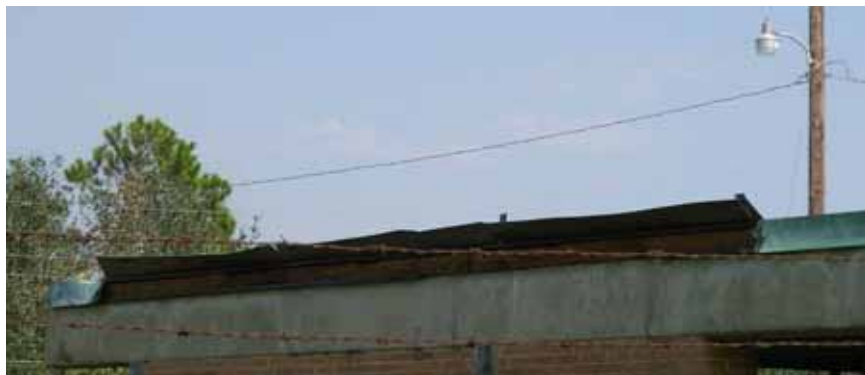
Figure 3-27 Example of perimeter metal flashing that was bent up and back from the building but without damage to the membrane, Port Arthur, TX (Photo credit: NIST).
