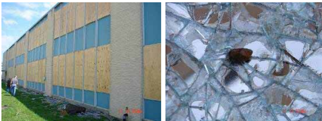
Figure 3-47 Broken glass at Memorial Ninth Grade School in Port Arthur, TX. The gravel among the broken glass was consistent with that on the aggregate-surfaced roof adjacent to this school (Photo credit: Jon Heintz, Applied Technology Council).
