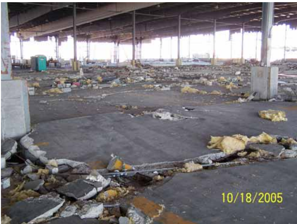
Figure 4-63 East Pier, showing damage to cargo shed deck and sheet metal siding (photo credit: Thomas B. Rodino, Shiner Moseley and Associates, Inc.)
