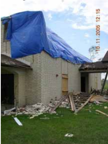
Figure 3-42 Failure of the windward, wooden truss in a recreation center in Port Arthur, TX (Photo credit: NIST).
