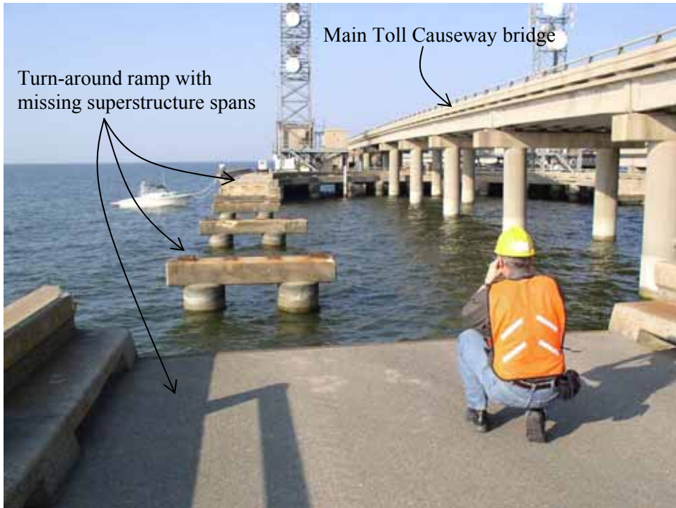
Figure 4-34 Toll Causeway turnaround bridge ramp failures (photo credit: Ron T. Eguchi, ImageCat).
