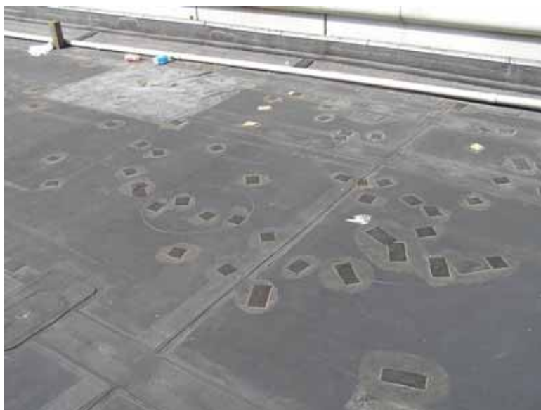
Figure 3-30 Adhered EPDM membrane system in New Orleans. The membrane was punctured by unknown wind-borne debris (Photo credit: Robb Smith, Amtech Roofing Consultants).
