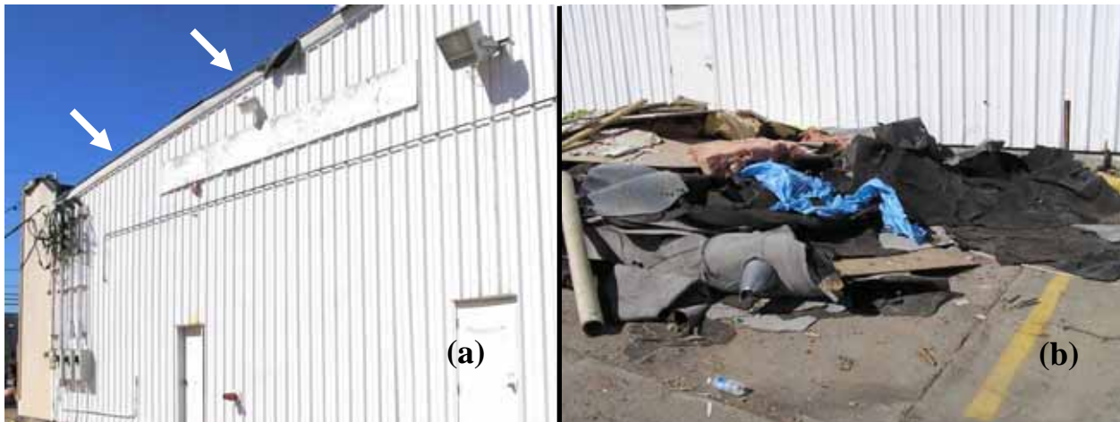
Figure 3-29 A commercial metal building in New Orleans that suffered damage to its modified bituminous membrane roof likely 15 as a result of insufficient fastening to the deck. Note in (a) damage to the edge detail (arrows). Note in (b) the debris pile, found below the damaged edge detail, containing sections of a modified bituminous membrane (Photo credit: Robb Smith, Amtech Roofing Consultants).
