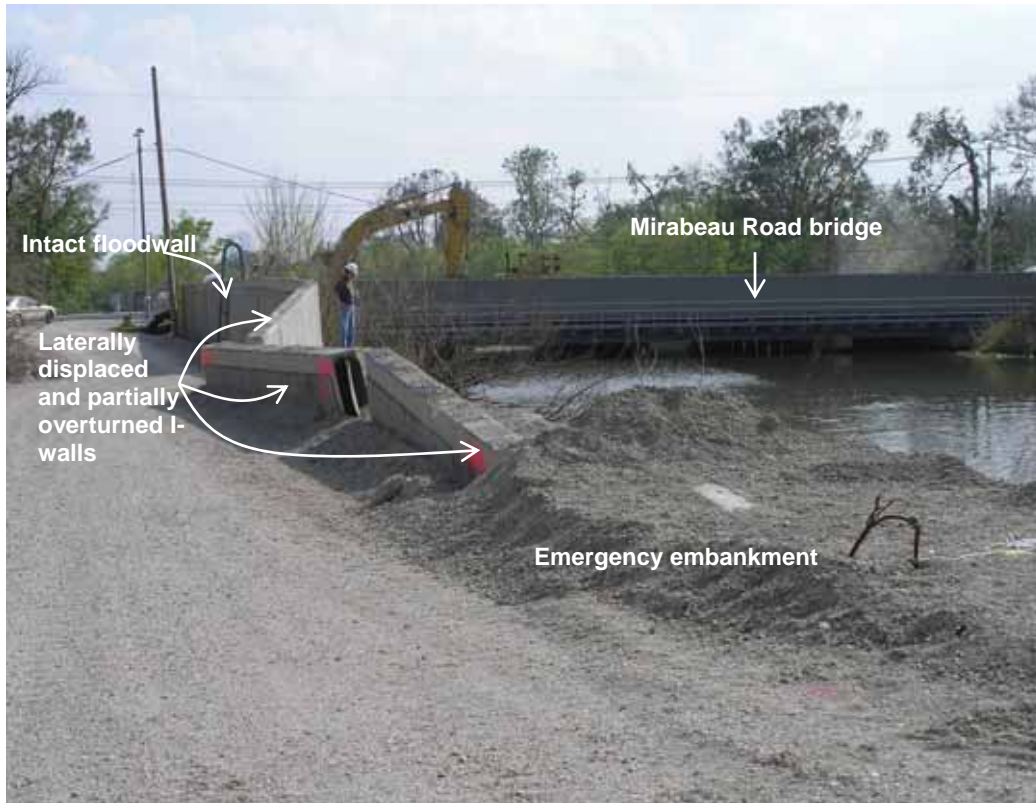
Figure 4-12 View looking south from the breach on the east bank of the London Avenue Outfall Canal toward Mirabeau Road bridge (photo credit: NIST)
