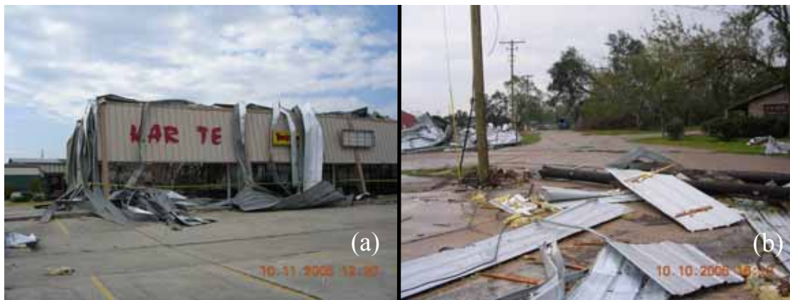
Figure 3-39 Failure of metal roofs in (a) Port Arthur, TX, and (b) West Orange, TX (Photo credit: NIST).
