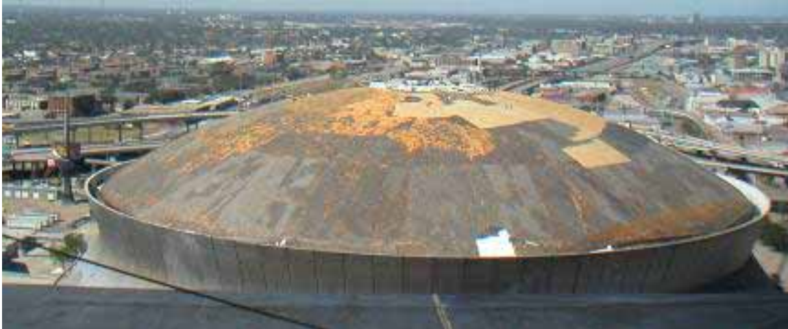
Figure 3-31 Louisiana Superdome. Gray areas are remaining polyisocyanurate insulation with a gray/black facer. Rust color is the original sprayed polyurethane foam (SPF). Tan is new SPF. The white area is a small section of white coated EPDM membrane that was not blown off. Before Hurricane Katrina, only the white coated EPDM membrane would have been visible on the roof (Photo credit: NIST).
