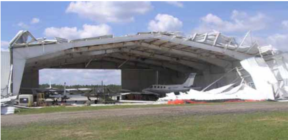
Figure 4-58 Hangar damage at Stennis Airport, Mississippi (photo credit: NIST)
