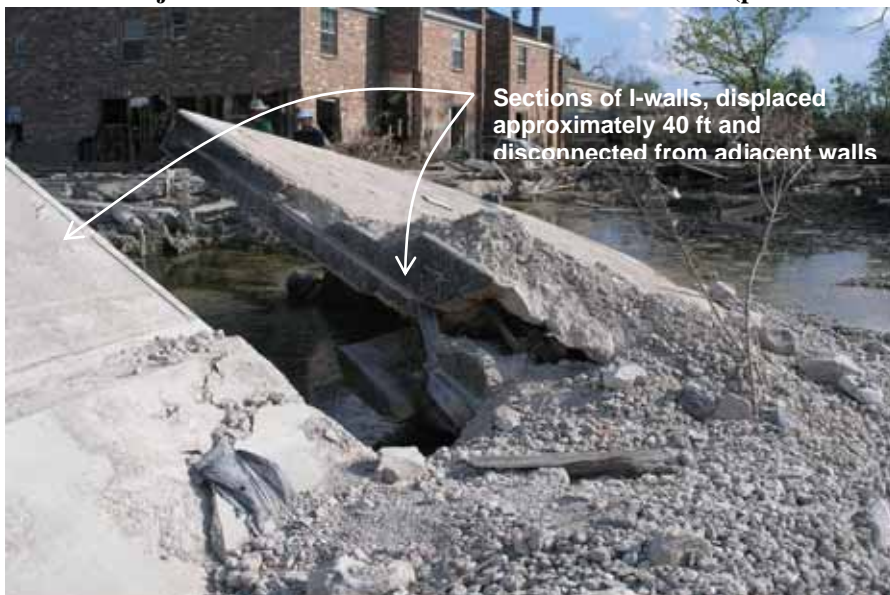
Figure 4-6 Sections of concrete I-walls displaced and disconnected from each other and from the steel sheet piles (photo credit: NIST)
