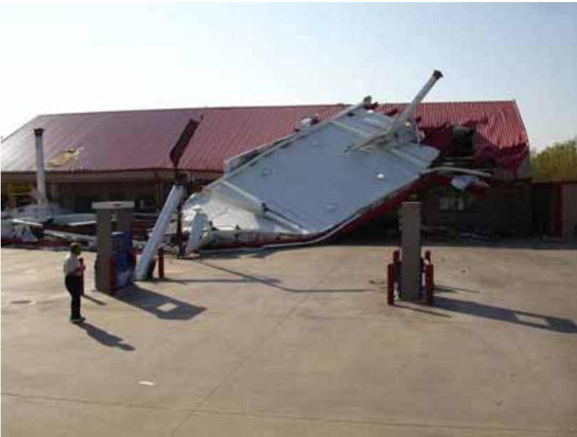
Figure 4-82 Gas station canopy near Port Arthur, Texas pulled out of its foundation (photo credit: NIST)
