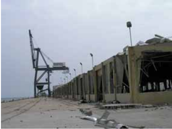
Figure 4-59 Damaged warehouse at Port of Gulfport (photo credit: NIST)
