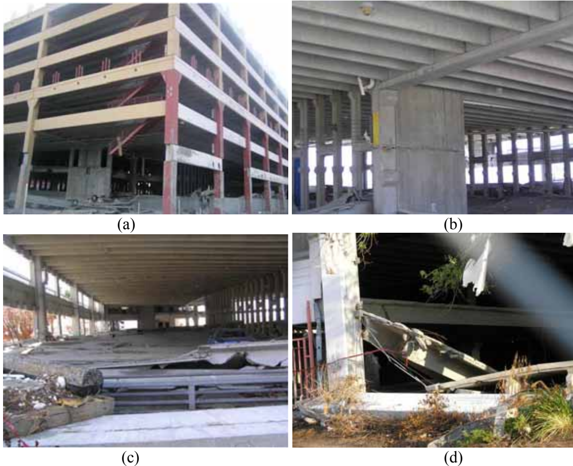
Figure 3-1 Partial, first-level collapse of precast, prestressed double-tee deck parking structures in (a) Gulfport, MS and (b,c,d) Biloxi, MS (Photo credit: NIST).
