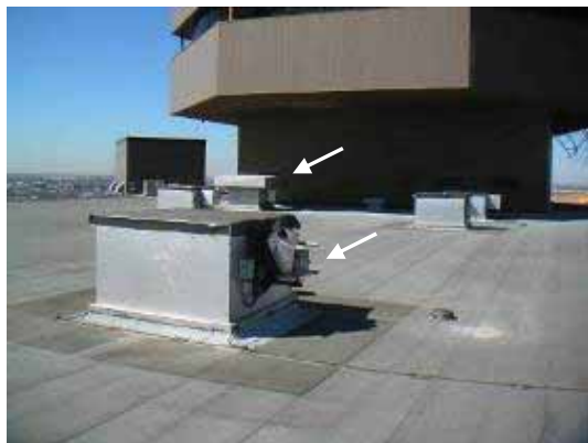
Figure 3-43 Five of six vents on the roof of the New Orleans Hyatt Regency were missing their hoods. Note the remaining hood in the background (arrow) and the missing cover of the fan motor of the vent in the foreground (arrow) (Photo credit: Keith Porter, Scawthorn Porter Associates).
