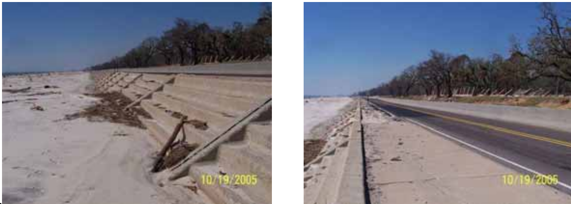
Figure 4-55 Seawall along US-90 protected much of the pavement from being undermined and washed out (photos credit: J. O'Connor, MCEER).
