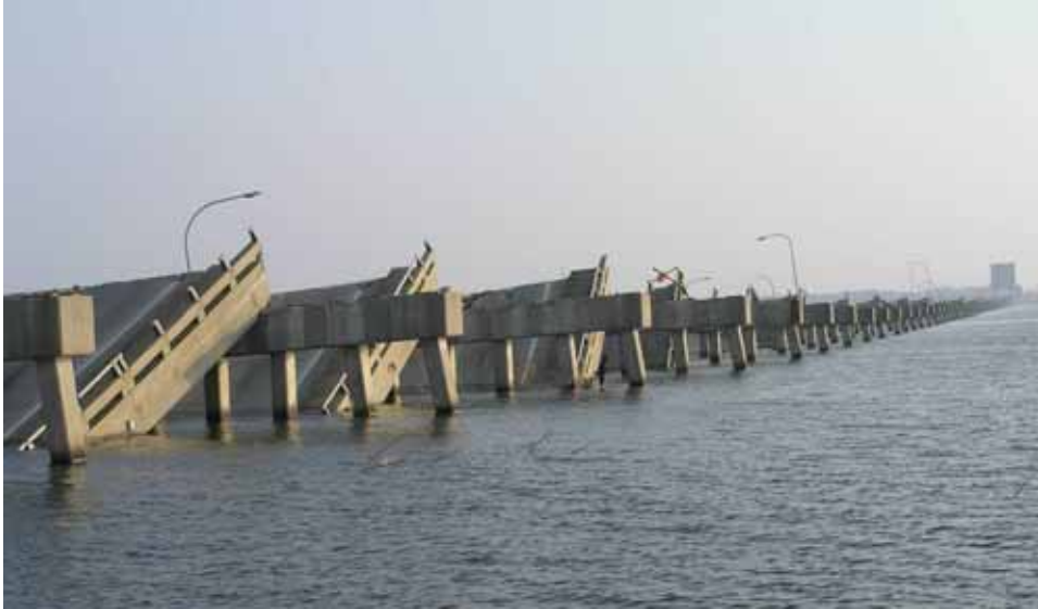
Figure 4-42 Looking west toward Biloxi from the east shore, many superstructure spans of US-90 Biloxi-Ocean Springs bridge were displaced north off their piers (photo credit: J. O'Connor, MCEER).
