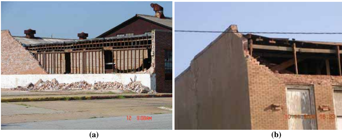
Figure 3-12 Failure of masonry parapet walls along the roof of buildings in Port Arthur, TX, (a) subsequent partial failure of exterior wall, (b) subsequent collapse (Photo credit: Jon Heintz, Applied Technology Council).
