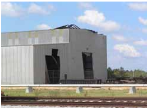
Figure 3-14 Permanent deformation of the windward wall inward and buckled purlins observed at the Port Bienville Industrial Park (Photo credit: NIST).
