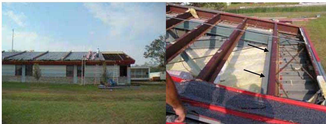
Figure 3-40 Missing roof clips (arrows) at the right eave of the Belle Chasse Middle School in Belle Chasse, LA. No evidence was seen that the clips had ever been installed (Photo credit: Robb Smith, Amtech Roofing Consultants).
