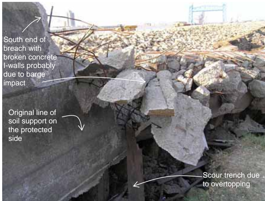
Figure 4-27 South edge of breach with broken concrete I-walls apparently 15 due to barge impact (photo credit: NIST)
