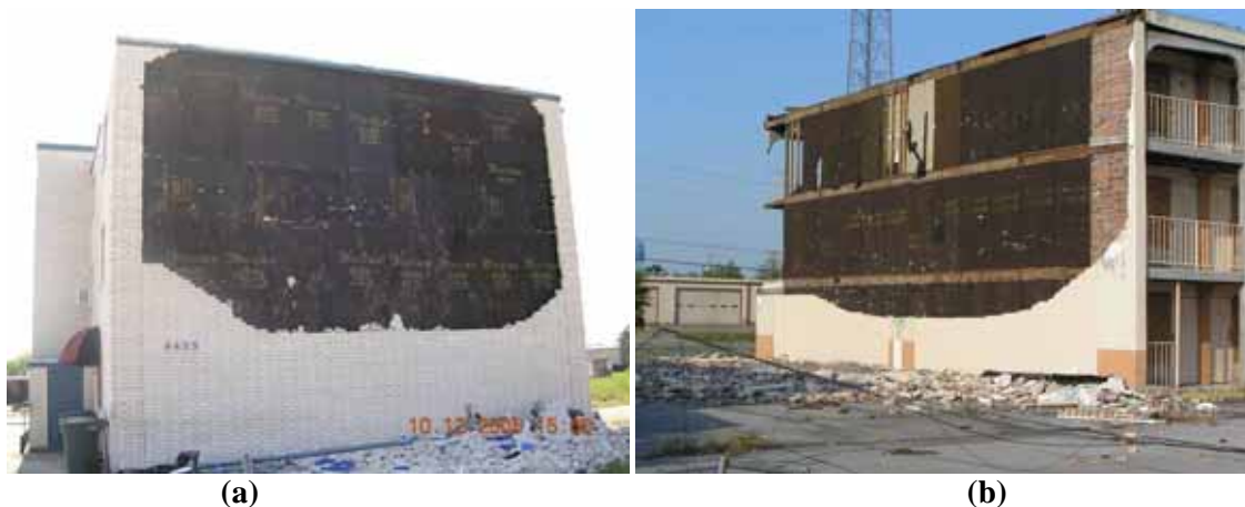
Figure 3-50 Wind-induced collapse of (a) a roughly 40 ft wide by 30 ft high and (b) a roughly 60 ft wide by 25 ft high, poorly anchored brick masonry cladding in Beaumont, TX (Photo credit: NIST).
