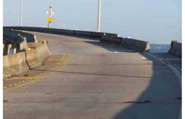
Figure 4-51 Bridge spans pushed north by the surge (photo credit: LA DOTD, provided by J. O'Connor, MCEER).
