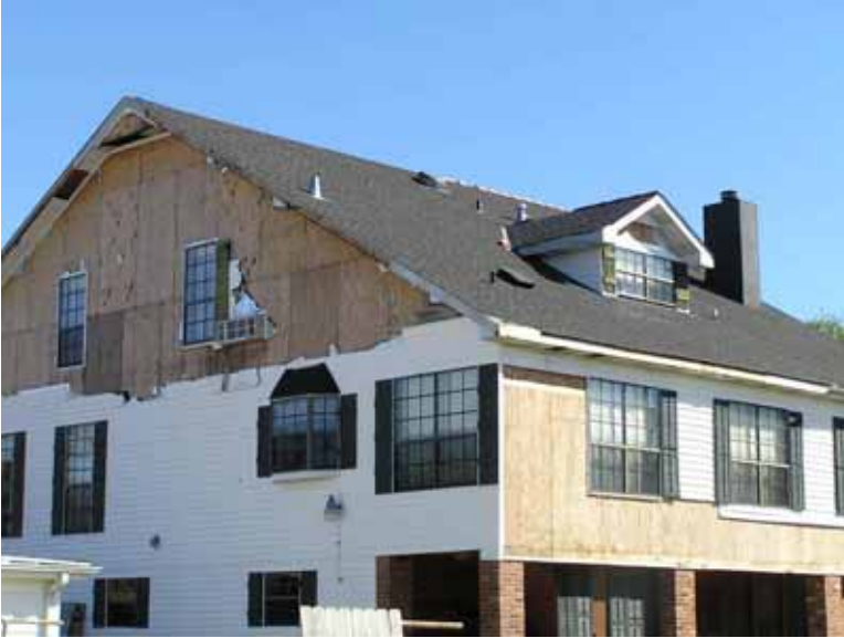
Figure 5-20 Damaged home where laminated asphalt shingles were intact; in contrast, considerable damage to vinyl siding and fascia boards occurred. This observation was not typical. In many cases and particularly in the Hurricane Rita impacted areas, homes not damaged by fallen trees, storm surge, or flooding often only sustained loss of roof coverings. Wall claddings, doors, and windows were often undamaged. (Photo credit: Robb Smith, Amtech Roofing Consultants)
