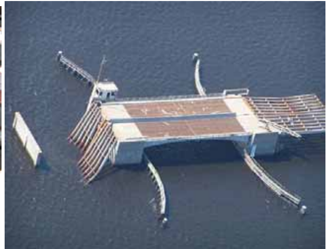
Figure 4-54 The lift spans of the US-90 bridge over St. Louis Bay became inoperable, blocking use of the channel by vessels (photo credit: J. O'Connor, MCEER).
