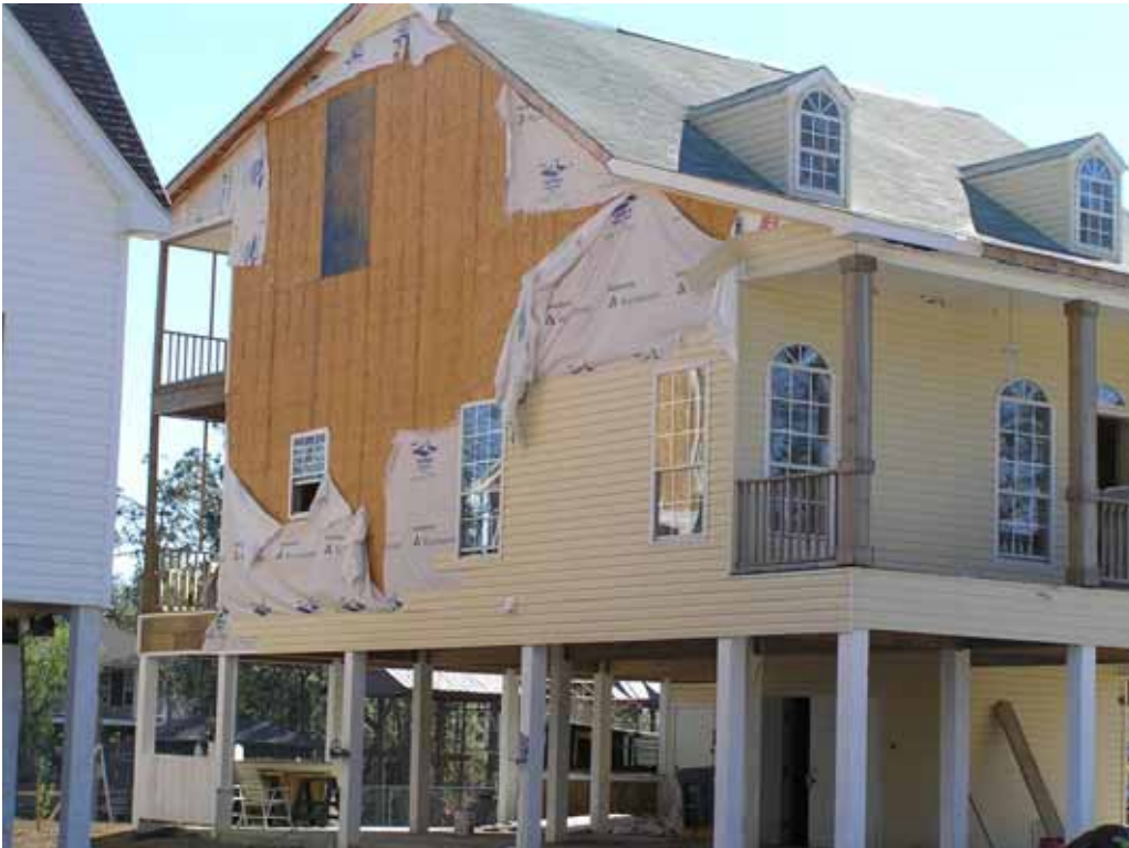
Figure 5-28 Damage to exterior cladding of a single-family residential structure near Pass Christian, Mississippi. (Photo credit: NIST)
