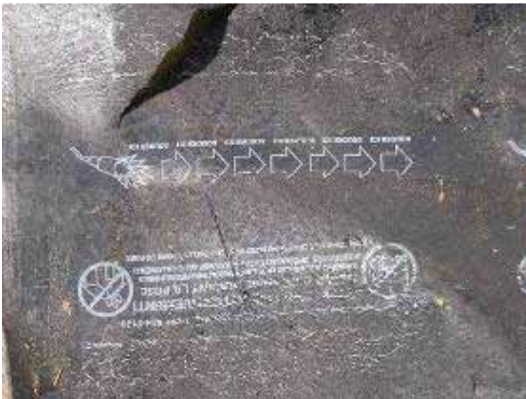
Figure 3-24 Had this failed heat bonded polymer-modified bitumen membrane been heated in accordance with acceptable practice, the plastic film and white markings would not be present (Photo credit: Robb Smith, Amtech Roofing Consultants).
