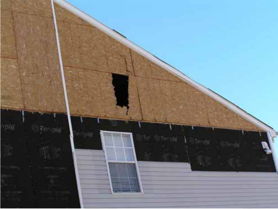
Figure 5-17 Damage to apartment building in Waveland, Mississippi due to wind-borne debris. (Photo credit: NIST)
