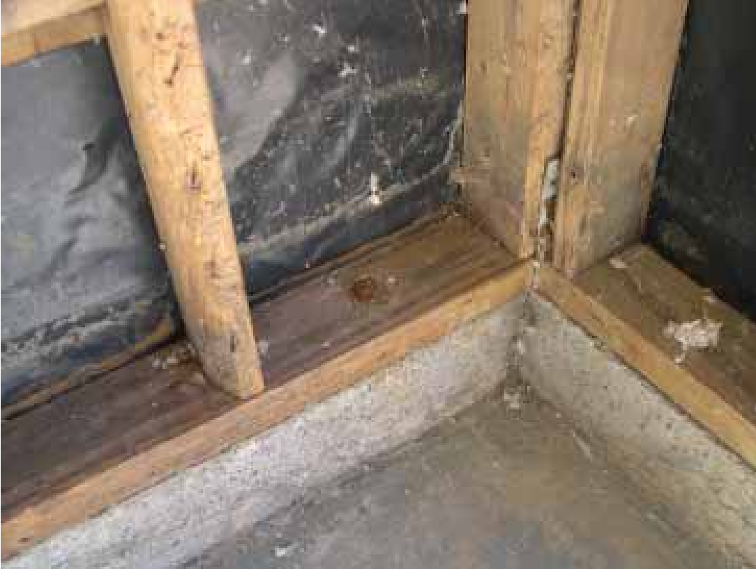
Figure 5-14 Walls anchored to the foundation remained intact. (Photo credit: Edwin T. Huston, Smith and Huston Inc.)
