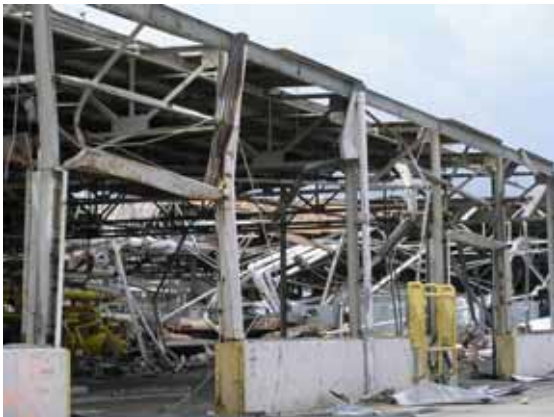
Figure 4-61 Damaged warehouse at Port of Gulfport, collapsed steel members (photo credit: NIST)
