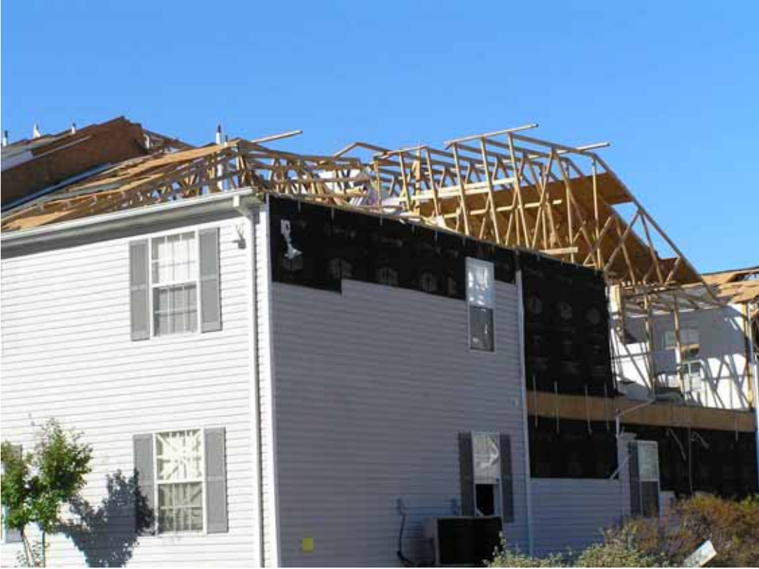
Figure 5-15 Wind damage to an apartment building in Waveland, Mississippi. (Photo credit: NIST)
