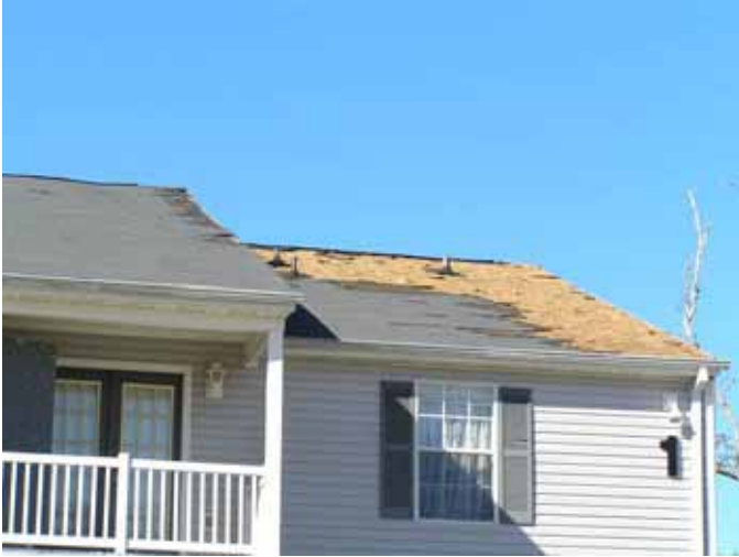
Figure 5-18 Loss of three-tab asphalt shingles where the underlayment was lost along with the shingles in New Orleans. Note the bare deck on the right. For many of the homes having damaged shingles, the underlayment or a previously installed shingle layer was in place, which may provide secondary backup against water penetration (photo credit: NIST).
