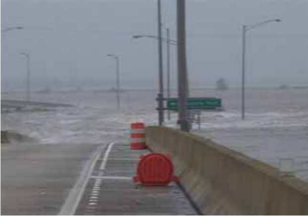
Figure 4-50 Surge waters overtopped US I-10 bridge ramp over Mobile Bay. View is eastbound, taken on the same day Hurricane Katrina hit (8/29/06). (Photo credit: George Conner, MSDOT)
