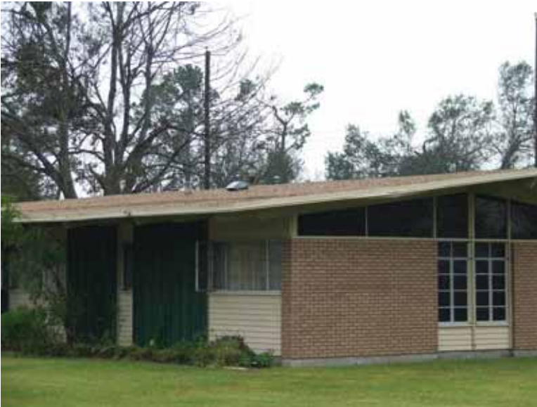
Figure 5-26 A small number of single-family, single-story homes having built-up bituminous membrane roofing (BUR) were seen. Those observed were undamaged as was the case for this house in Orange, Texas. (Photo credit: Dominic Sims, International Code Council)
