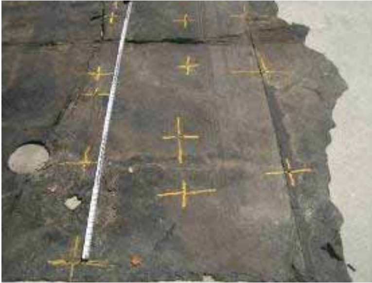
Figure 3-23 Irregularly spaced nailing on this failed hot-applied built-up roofing membrane had approximately 40 percent fewer nails than specified by a typical manufacturer (Photo credit: Robb Smith, Amtech Roofing Consultants).
