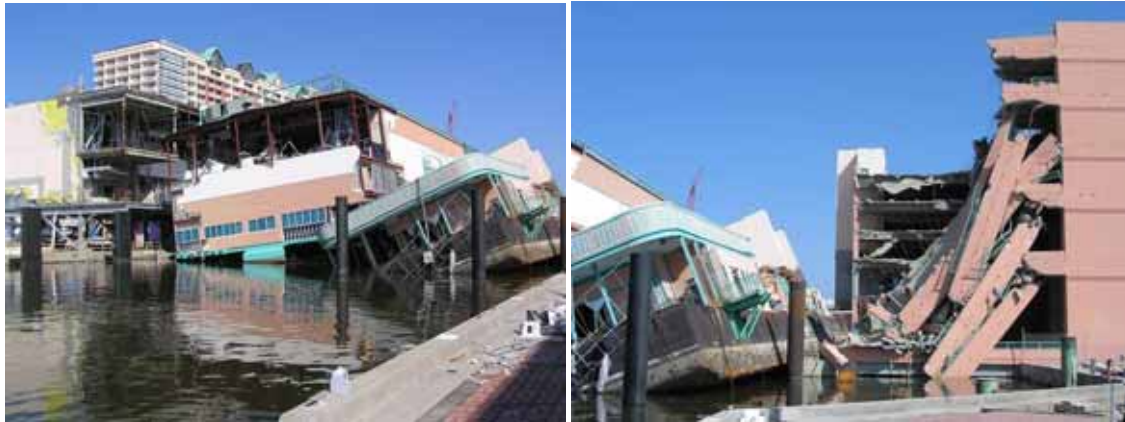
Figure 3-18 Partial collapse of a precast reinforced concrete garage due to impact by a Biloxi, Mississippi casino barge (Photo credit: NIST).
