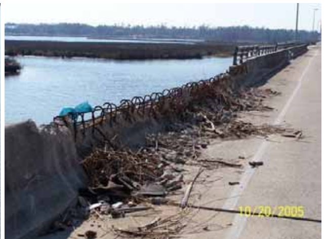
Figure 4-48 Broken curb rail, Popps Ferry bridge (photo credit: J. O'Connor, MCEER)
