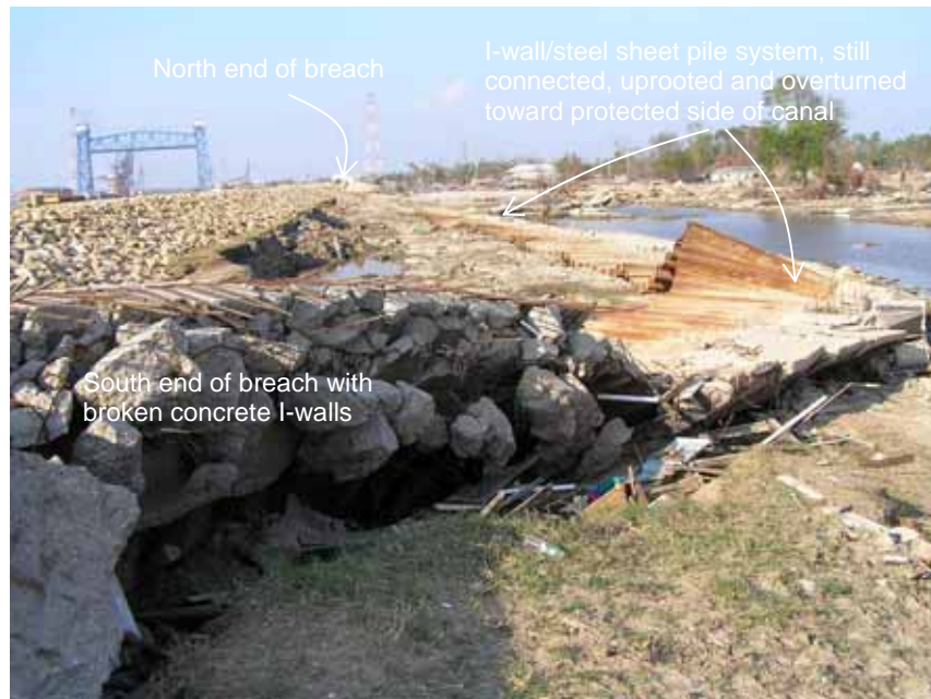
Figure 4-26 Overturned and uprooted floodwall at the IHNC Lower Ninth Ward South breach, with the I-walls remained connected to the sheet piles (photo credit: NIST)
