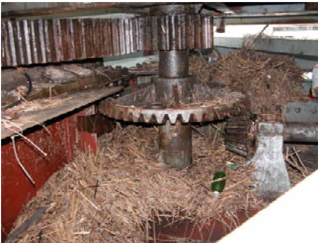
Figure 4-53 Typical debris buildup in the gear mechanism of a moveable bridge (photo credit: LA DOTD, provided by J. O'Connor, MCEER).
