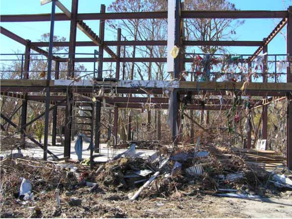
Figure 5-8 Coastal residential structure with steel-frame skeleton and in-fill wood framing West of Bay St. Louis, Mississippi. The steel frame survived, but the in-fill wood framing was destroyed. (Photo credit: NIST)
