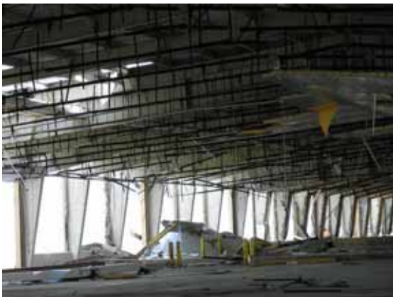
Figure 4-60 Damaged warehouse at Port of Gulfport, with steel frames still standing (photo credit: NIST)
