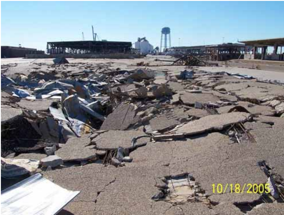
Figure 4-62 West Pier, showing collapse of wharf structure due to pile failure (photo credit: Thomas B. Rodino, Shiner Moseley and Associates, Inc.)
