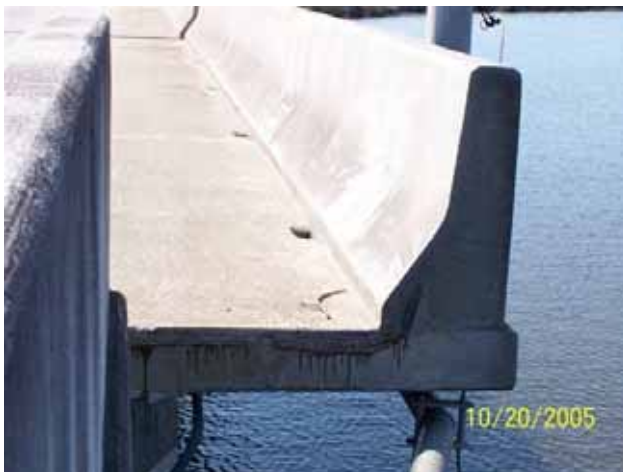
Figure 4-47 Displaced spans of Popps Ferry Bridge (photo credit: J. O'Connor, MCEER)
