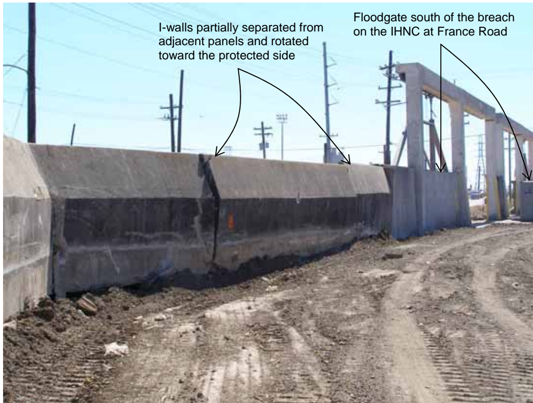
Figure 4-18 View from the protected side looking south from the breach showing distressed I-walls adjacent to floodgate on IHNC at France Rd (photo credit: NIST)
