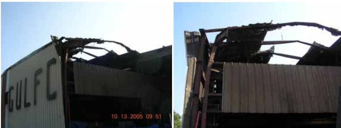
Figure 3-16 Buckled purlins and collapse of a portion of the end bay of a steel-frame warehouse from wind pressure in Beaumont, TX (Photo credit: NIST).
