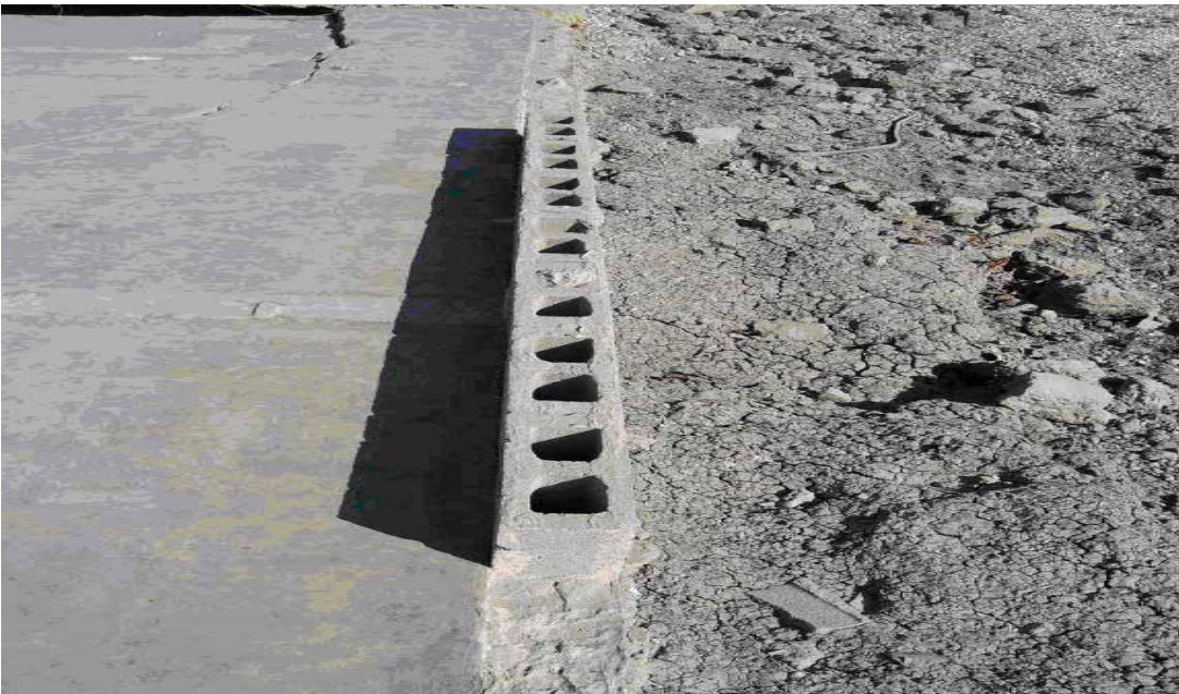
Figure 5-13 Typical foundation in New Orleans showed lack of anchor bolts. (Photo credit: Edwin T. Huston, Smith and Huston, Inc.)
