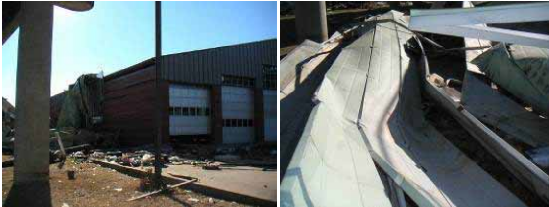
(a) (b) Figure 3-38 New Orleans Third District Fire Headquarters. (a): roof damage. (b): apparent lack of fasteners (Photo credit: Keith Porter, Scawthorn Porter Associates).
