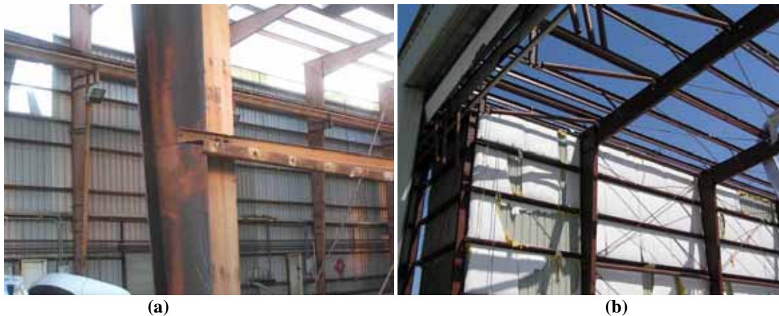
Figure 3-36 Loss of corrugated-metal roofing structures on large, metal buildings in a) Pass Christian, MS, and b) Port Arthur, TX (Photo credit: NIST).
