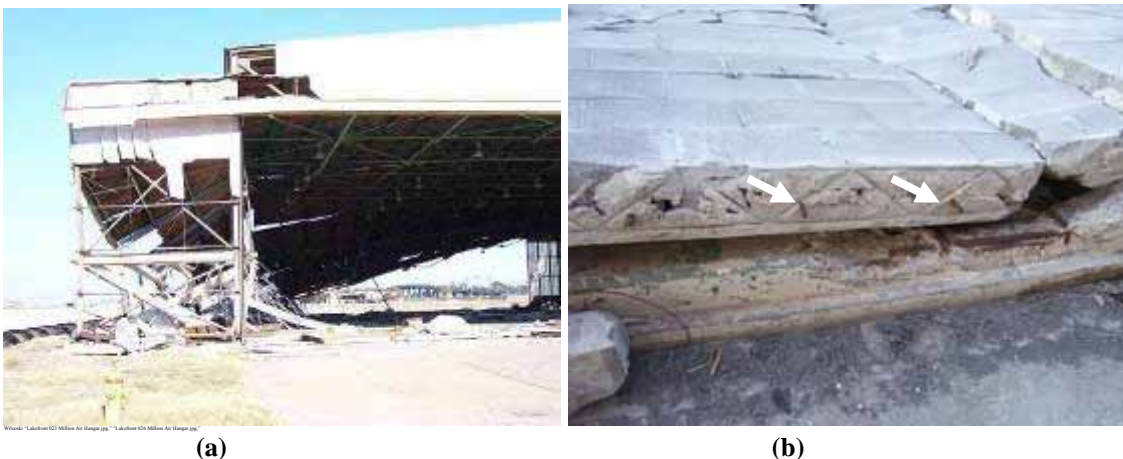
Figure 3-8 (a): Partial collapse of aircraft hangar apparently 15 as a result of the collapse of a CMU infill wall. (b): 3 in lap splice at base of collapsed CMU wall (Photo credit: Ed Huston, Smith and Huston, Inc.)
