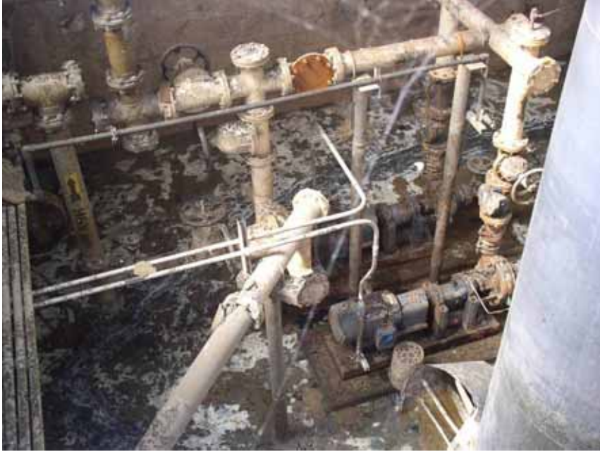
Figure 4-75 Eastbank Wastewater Treatment Facility. Damaged pumps in lower right-hand corner. Facility was under water for approximately three weeks (photo credit: Ron T. Eguchi, ImageCat)
