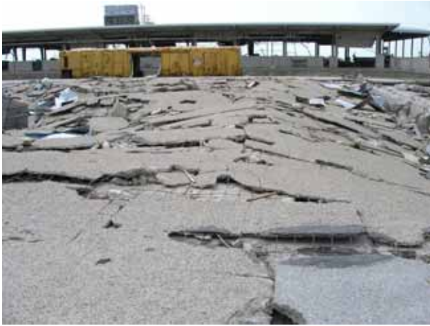
Figure 4-64 Wharf buckled upward due to storm surge pressure (photo credit: Thomas B. Rodino, Shiner Moseley and Associates, Inc.)
