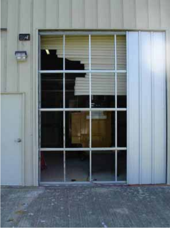
Figure 4-73 Roller door failure (with temporary framing and cladding) that led to auxiliary generator shutdown at Central Water Treatment Plant in Beaumont, Texas (photo credit: Christopher Letchford, Texas Tech University)
