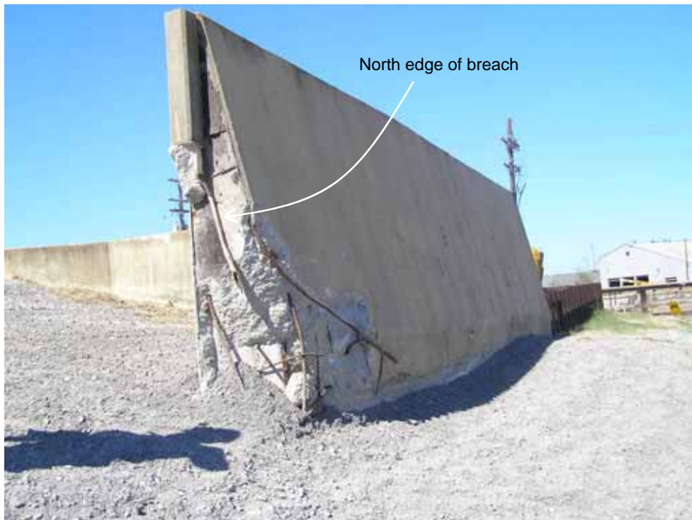
Figure 4-23 View looking north at the north edge of the IHNC Lower Ninth Ward North breach (photo credit: NIST)
