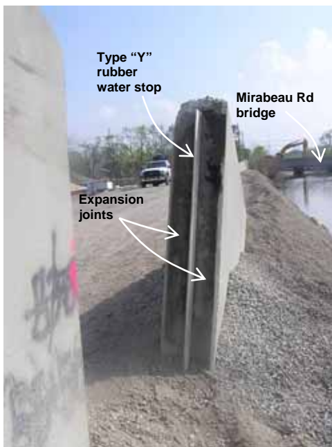
Figure 4-13 I-walls of failed floodwall section separated along water stop joint (photo credit: NIST)
