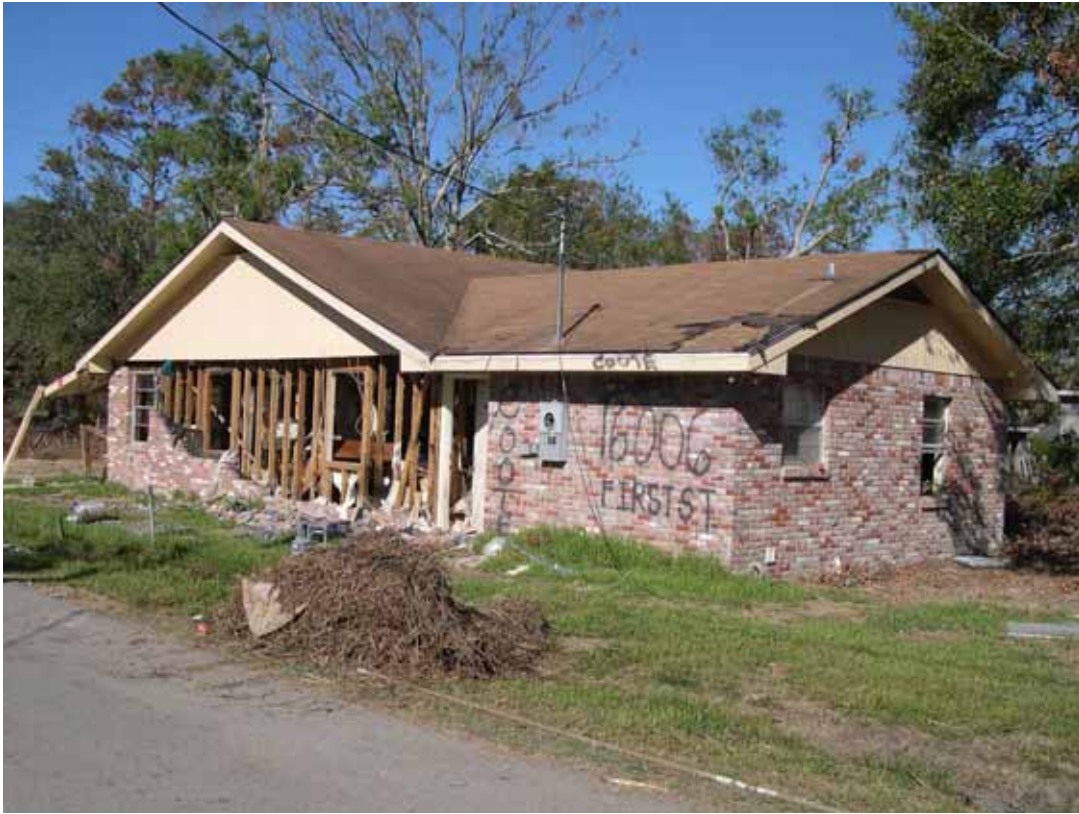
Figure 5-29 Damage to brick cladding and other exterior wall components for a single-family dwelling in Pearlington, Mississippi. (Photo credit: Jay H. Crandell, Applied Residential Engineering Services)
