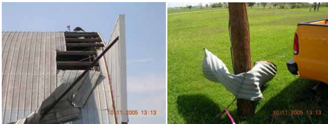
Figure 3-37 Damaged metal panels on a barrel roof at the Southeast Texas Regional Airport, Port Arthur, TX (Photo credit: NIST).
