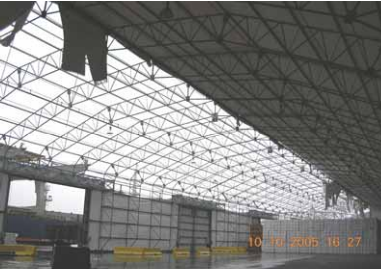
Figure 4-68 Fabric roof failure on warehouse, Port of Port Arthur, Texas (photo credit: NIST)
