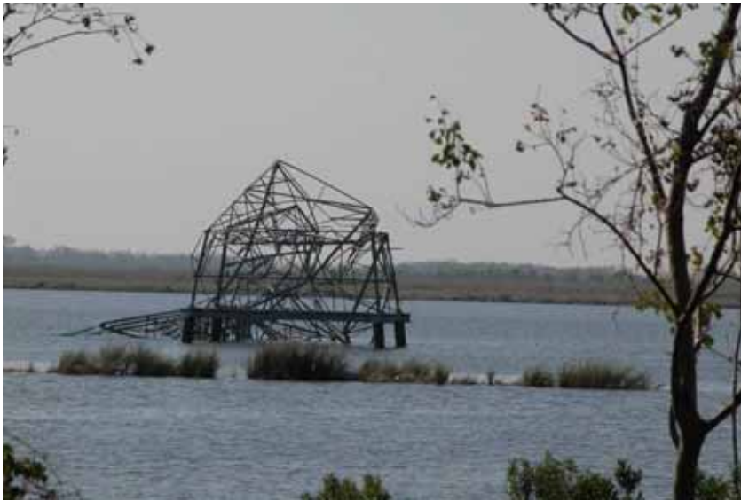
Figure 4-70 Failure of transmission line lattice tower on the Neches River (Ocean Springs to Moss Point) near Bridge City, Texas following Hurricane Rita (photo credit: NIST)
