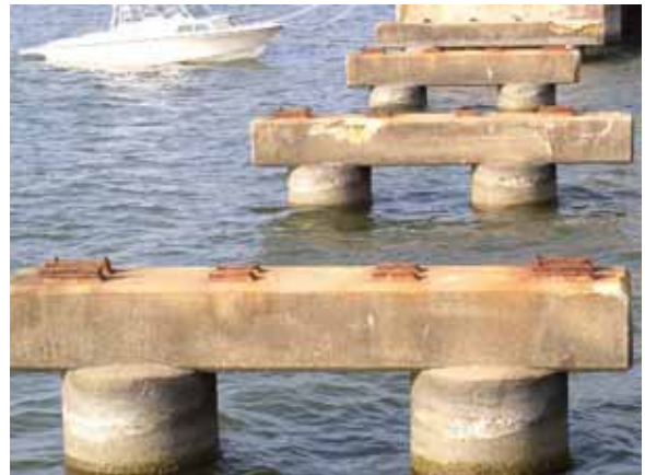
Figure 4-36 Steel Bearing Plates/Shear Keys connection between the superstructure and the bridge piers (photo credit: Ron T. Eguchi, ImageCat)
