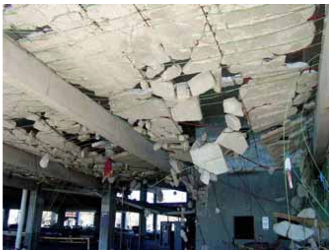
Figure 3-3 Failure of post-tensioned concrete slab exposed to uplift forces due to storm surge (Photo credit: Jack Hayes, USACE)
