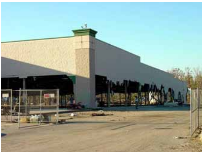
Figure 3-5 Storm-surge-induced collapse of the lower portions to a reinforced CMU wall in Gulfport, MS (Photo credit: Habib Rahman, National Research Council of Canada).
