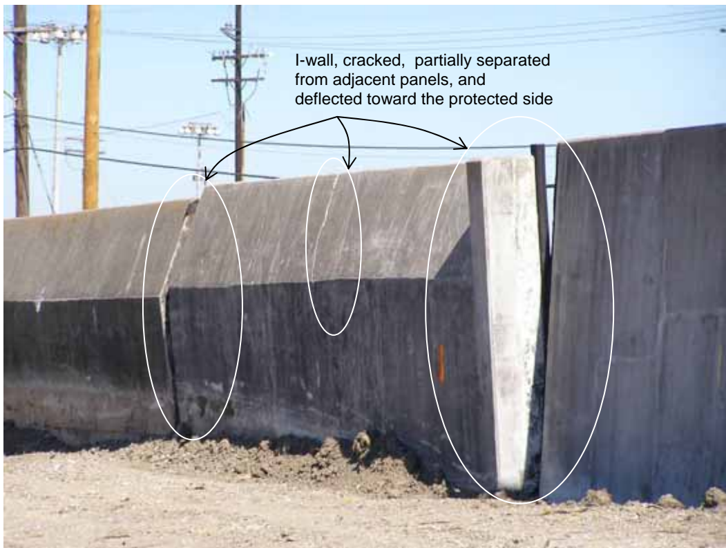
Figure 4-19 View from the protected side south of the breach showing distressed I-walls near the floodgate on IHNC at France Rd. (photo credit: NIST)
