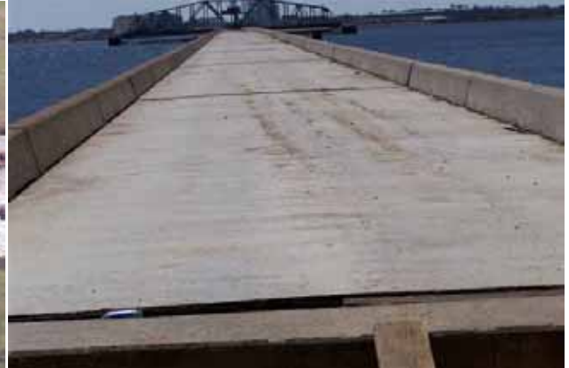
Figure 4-57 CSX railroad bridge over Biloxi Bay after tracks and ties were washed off by storm surge and wave action (photo credit: J. O'Connor, MCEER)
