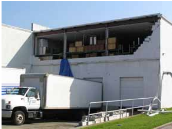
Figure 3-9 Failure of a non-load bearing masonry wall in Beaumont, TX (Photo credit: NIST).
