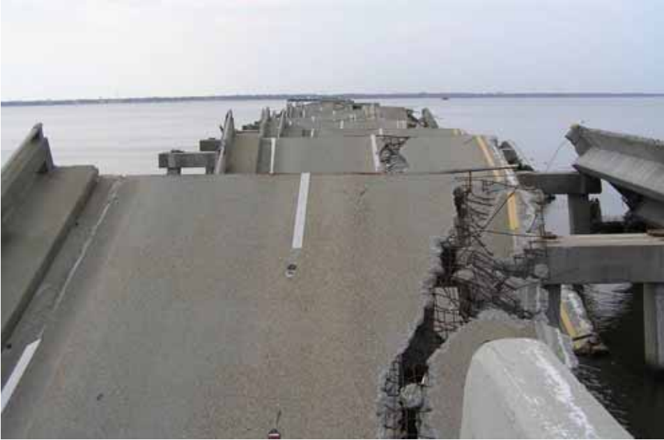
Figure 4-38 Displaced and dropped superstructure spans of US-90 bridge over St. Louis Bay (photo credit: NIST).
