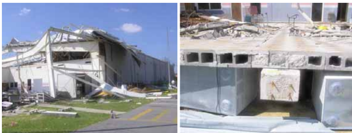
Figure 3-10 Damage to Gaston Hewes Recreation Center in Gulfport, Mississippi (Photo credit: NIST).
