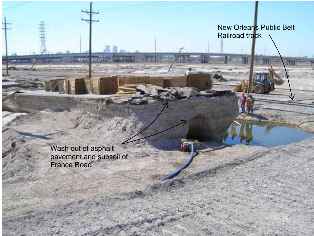
Figure 4-20 Erosion due to scour at France Road at section south of the breach in the floodwall on the west bank of the IHNC (photo credit: NIST)
