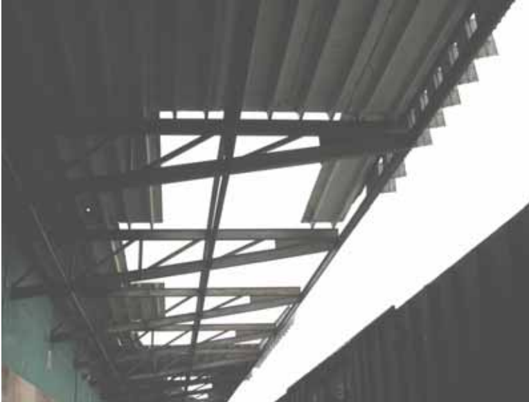
Figure 4-67 Concrete double-T beam blow-off on warehouse overhang, Port of Port Arthur, Texas (photo credit: NIST)
