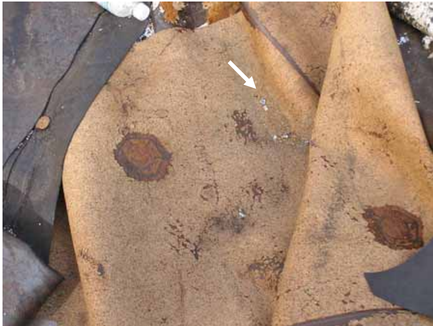
Figure 3-32 Section of damaged EPDM membrane found on the roof of a building downwind from the Superdome. The tan color represents adhesive used to attach the EPDM to the insulation on the Superdome. The white specs (arrow) are pieces of broken glazing from windows of a nearby building that was also downwind from the Superdome (Photo credit: Robb Smith, Amtech Roofing Consultants).
