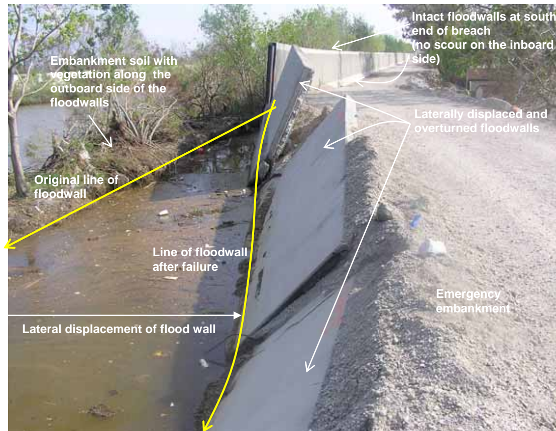
Figure 4-8 View looking south of the breach on the west bank of the London Avenue Outfall canal near Robert E. Lee Road (photo credit: NIST)
