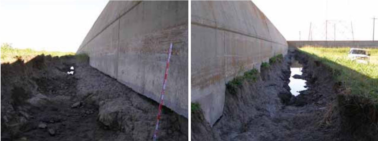
(a) (b) Figure 4-29 Scour trench along floodwall next to Entergy Michoud Power Plant (photo credit: NIST).
