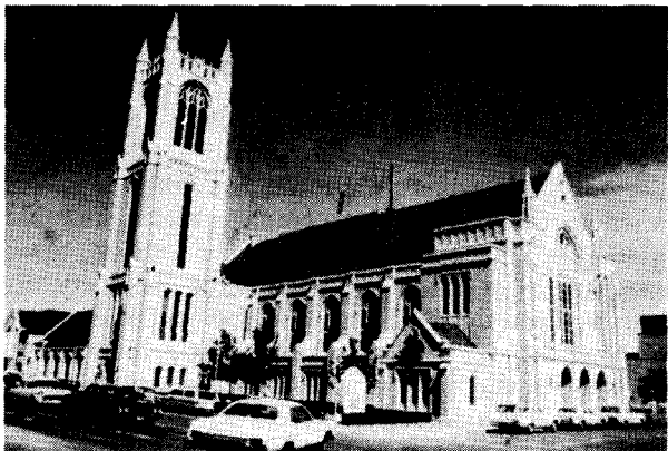
Photograph 17—View of First Methodist Church looking northwest. This masonry structure sustained only minor damage to clay roof tiles and to glazing. (Location 10)
