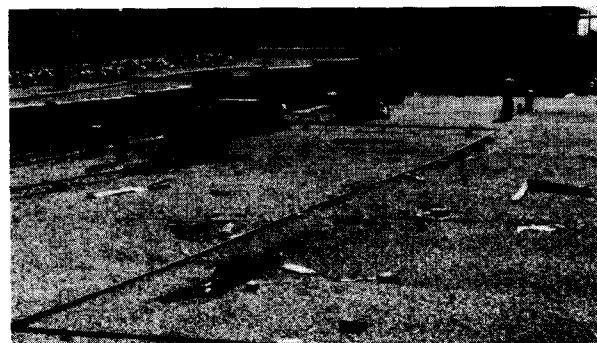
Photograph 31—View looking northeast showing roof of Recruiting Station for U.S. Military Services. Note punctured roof in foreground and overturned parapet wall to the rear. (Location 16)
