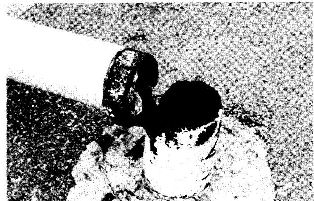
Photograph 15—Weld-fracture at base of sign posts shown in Figure 14. (Location 9)
