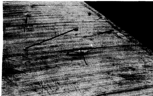
Photograph 64—Mobile home aluminum roof shows denting and splitting of seams caused by hailstone impact. (Location 34)
