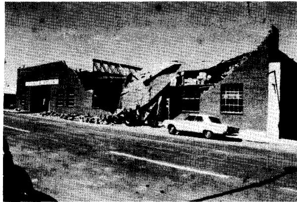
Photograph 18—Maintenance shops of Texas, New Mexico and Oklahoma Coach Company. View looking southwest. (Location 11)
