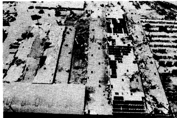
Photograph 39—Damage to roofs of light industrial buildings of the Hancock Division of Clark Equipment Company. View looking west. (Location 22)
