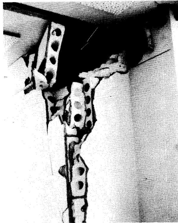
Photograph 23—Disruption of gypsum-tile fire protection to steel column in the Great Plains Life Building. (Location 13)
