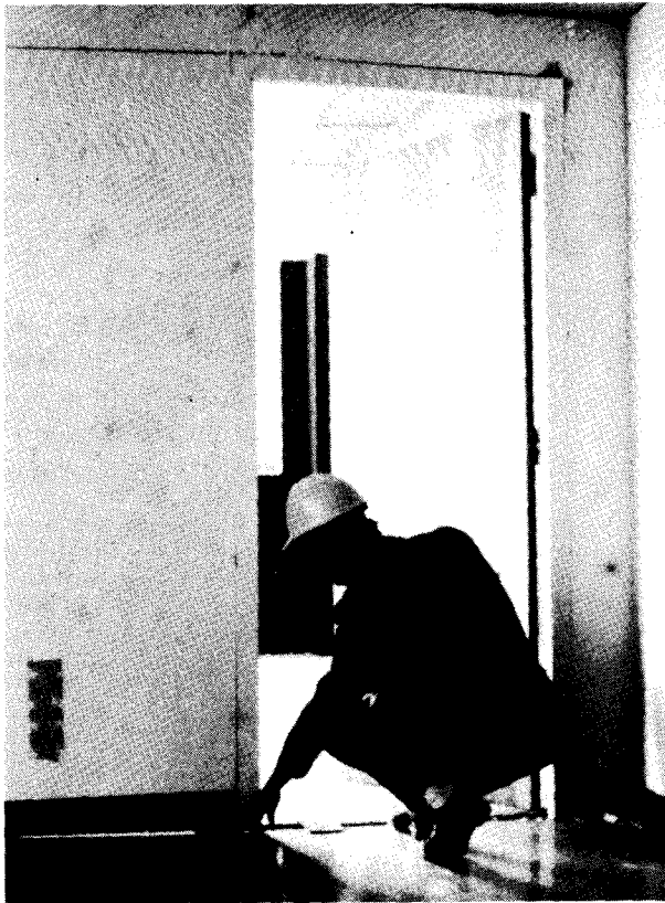
Photograph 25—One inch vertical movement of gypsum tile partition at southeast corner of sixth floor of Great Plains Life Building. Note racking of door frame. (Location 13)
