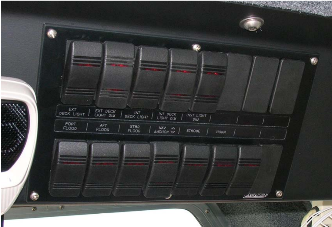
Figure 3-81 Light Switch Panel
