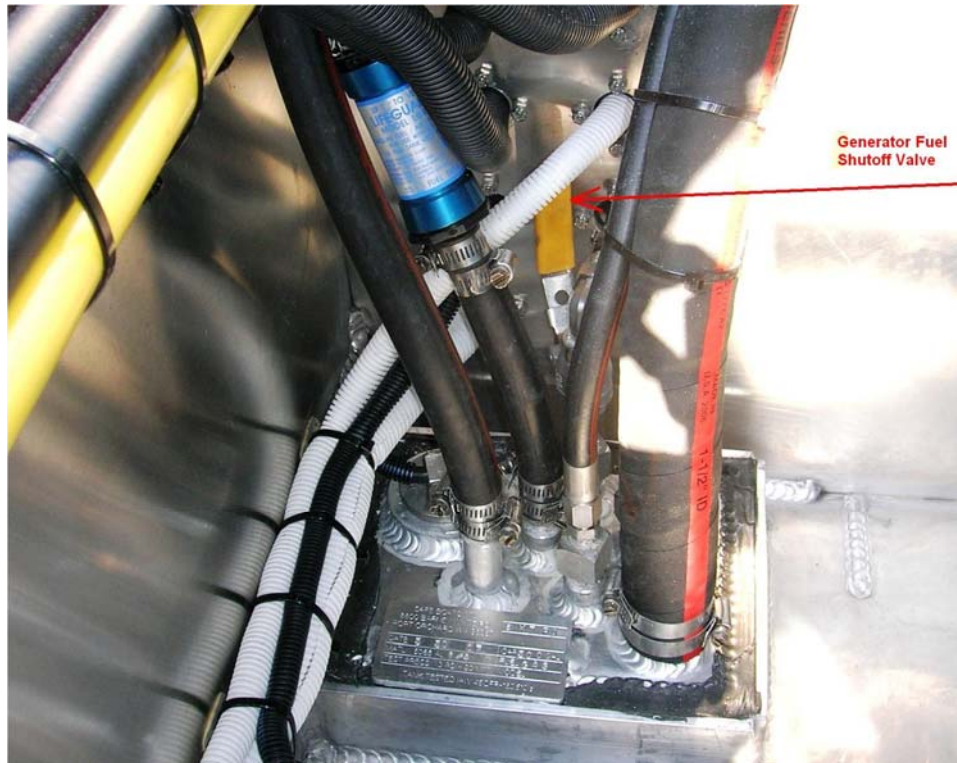
Figure 3-65 Generator Fuel Shutoff
