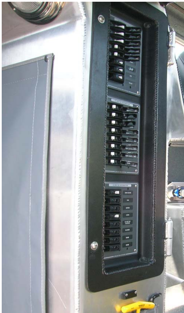
Figure 3-59 12 VDC Distribution Panels
