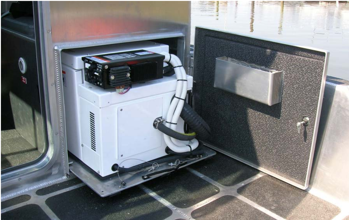
Figure 2-13 Generator Compartment with Access Panel Open
