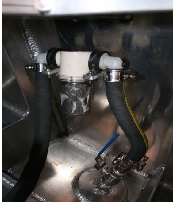
Figure 3-64 Generator Cooling Water Piping
