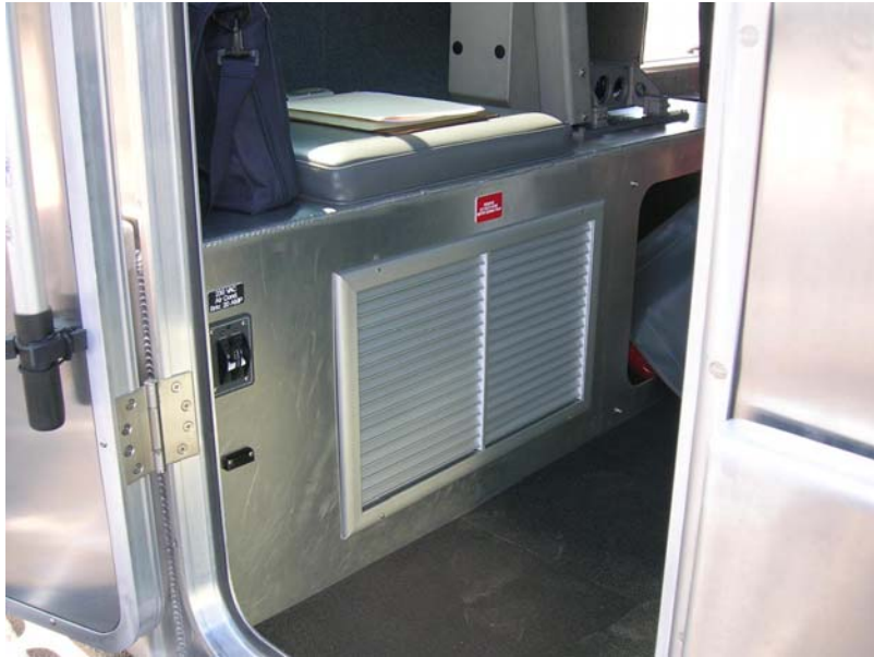
Figure 3-71 Heat and A/C 20 amp Breaker
