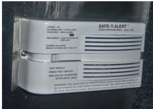
Figure 3-94 Carbon Monoxide Detector
