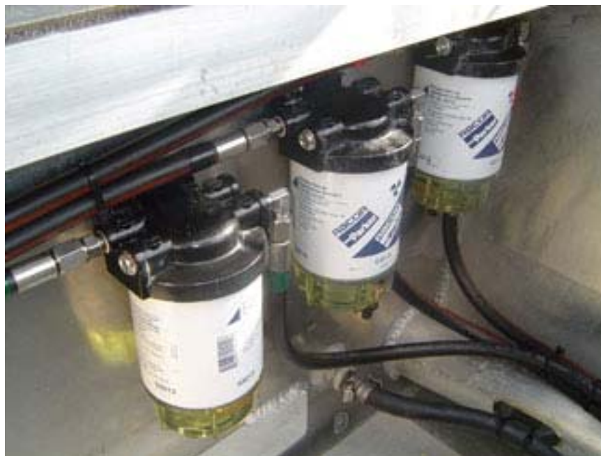
Figure 2-33 Fuel Filters in Port Aft Deck Locker
