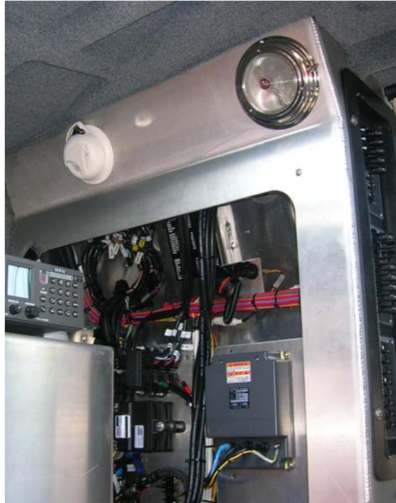
Figure 3-60 Console Wiring Access
