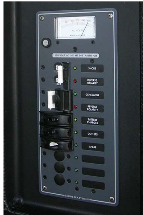
Figure 3-68 AC Power Distribution Panel
