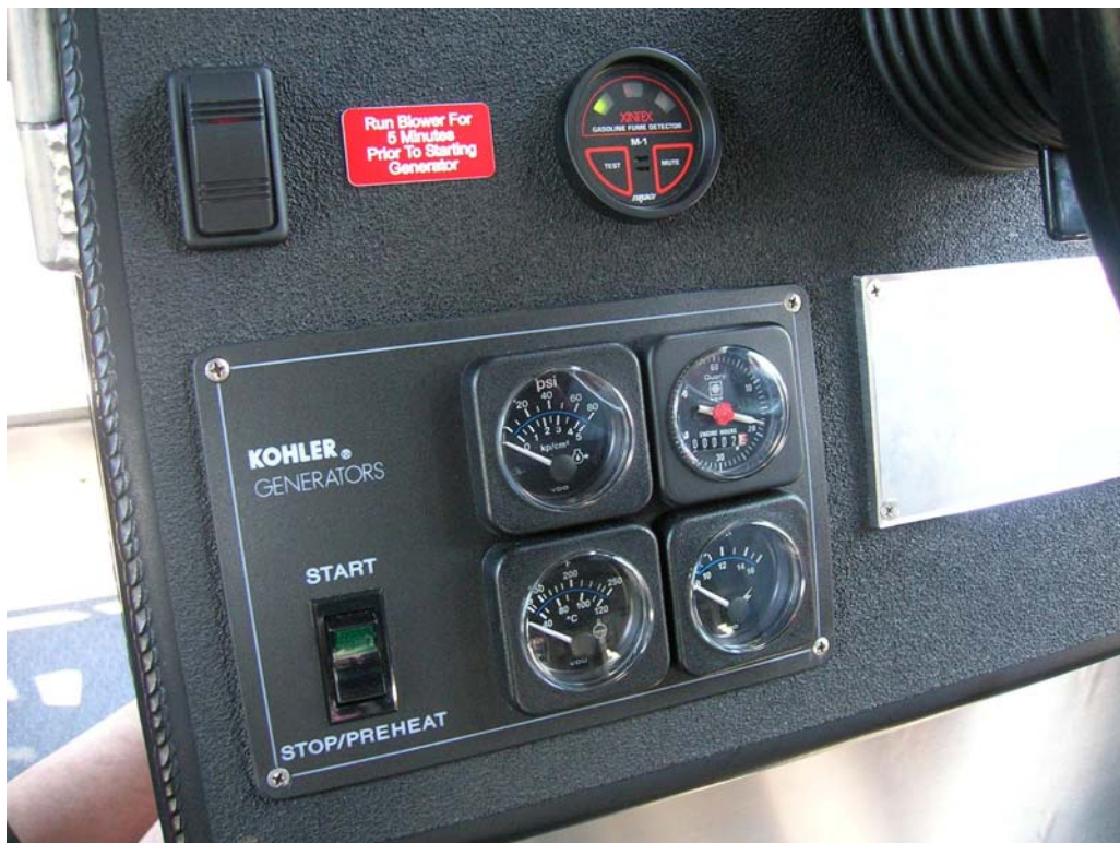
Figure 3-62 Generator Control Panel
