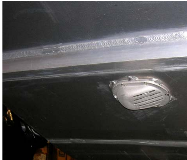
Figure 2-15 Seawater Suction Seachest Strainer
