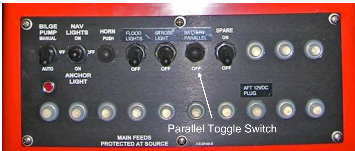
Figure 3-37 Switches and Circuit Breakers (Coxswain's Console)
