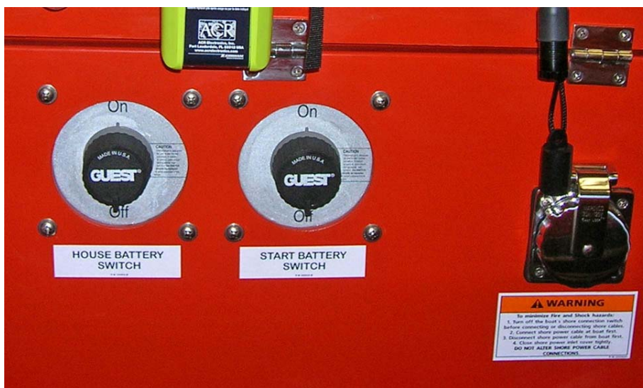
Figure 3-32 Battery Switch and Shore Power Connection
