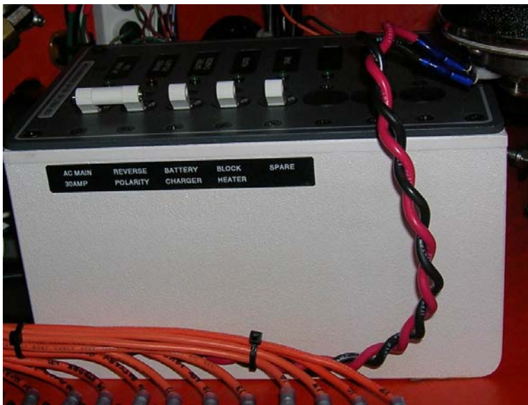
Figure 3-34 AC Breaker Panel
