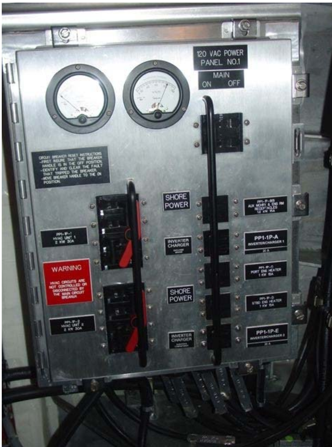
Figure 3-11 120 VAC Power Panel
