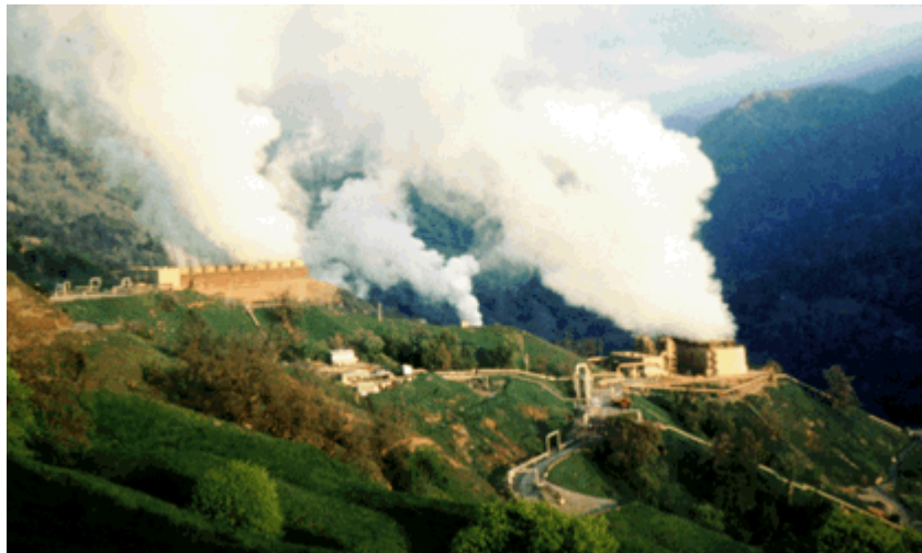
Geothermal powerplant at The Geysers near the city of Santa Rosa in northern California. The Geysers area is the largest geothermal development in the world. (Photograph by Julie Donnelly-Nolan, USGS.)
